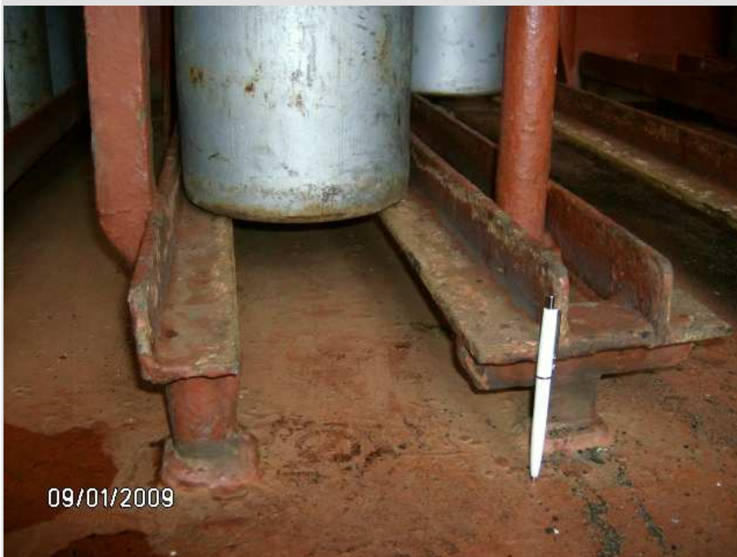
The bottom of CO 2 cylinders, not firmly standing in the racks
