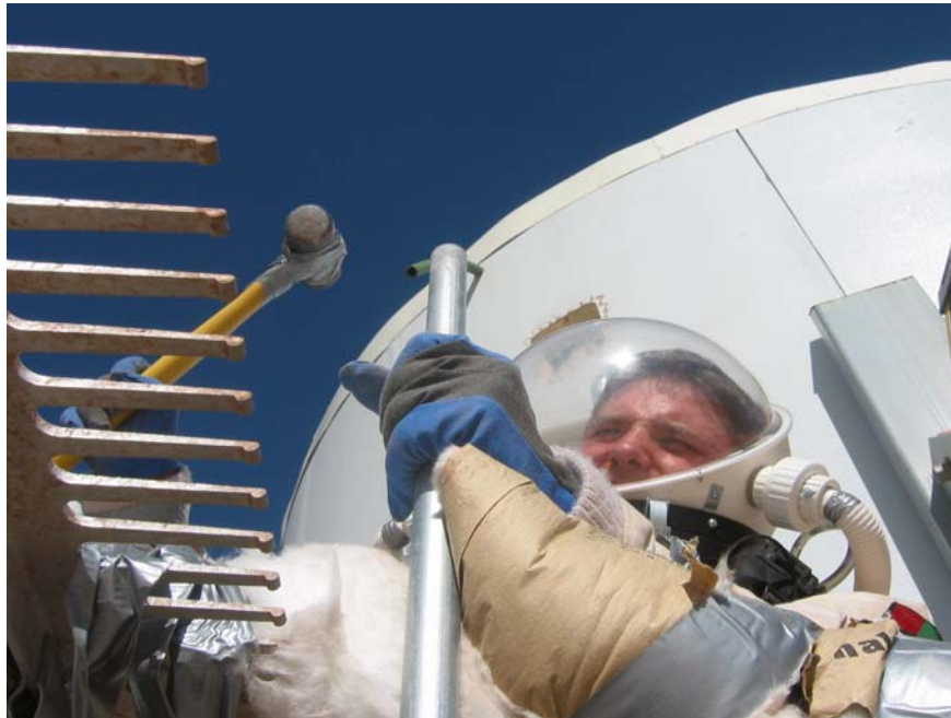
Fig. 1. Maintenance tasks will represent a considerable, ongoing burden for future Mars explorers, unless the workload can be reduced by robots. Here engineer Matt Bamsey repairs a collapsed water pipe support outside the Mars Desert Research Station, Utah during a 2003 simulation. .
