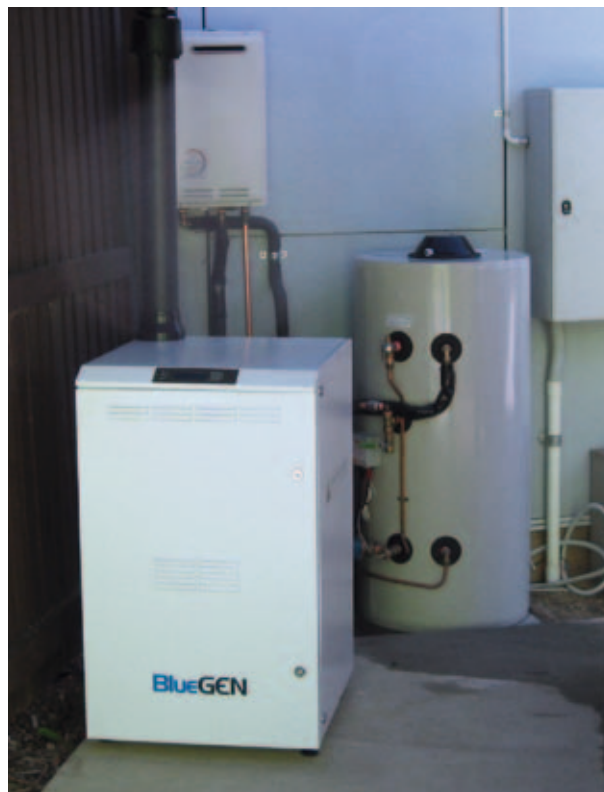
BlueGen installation at VicUrban's Aurora housing development in Epping, Melbourne.
