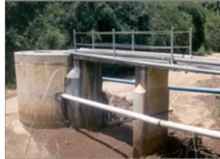
Figure 4.1 Collection well at Peyanar Headworks
