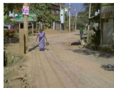
Fig 4.9: Link Road to Madurai Road for Town Buses – Severely Damaged
