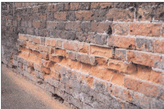
Pollution damage to brickwork in The Street
