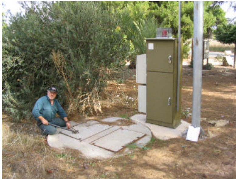
STEDS Maintenance Officer alongside pump station
