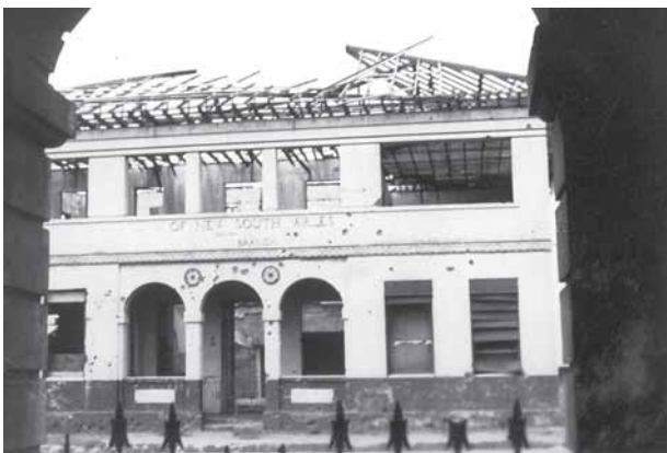
The remnants of the bombed Bank of New South Wales in Darwin, now the facade of the Westpac Bank in the Smith Street Mall.
