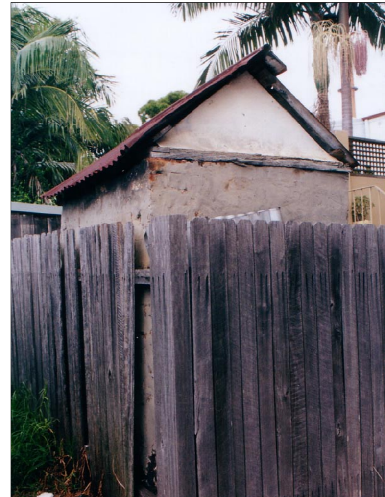
Fig 15.1 Last dunny in Green Square? A surviving outhouse in Green Square. Discovered by the HIST3904 class in Nevins Lane, at the rear of a terrace house in Portland Street, Zetland. (Photo: Grace Karskens 2004.)
