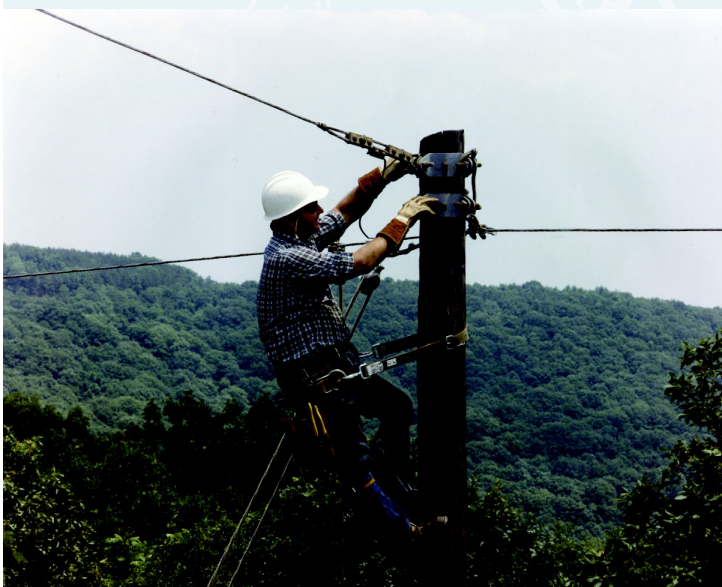
Line Crewman checking equipment near Springfield, Missouri.
