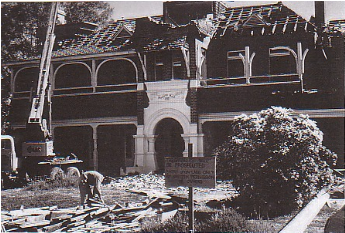
Photo 20: Demolition of Haddon Hall 1976. (Courtesy of KD Leach, Former City of South Perth Librarian)
