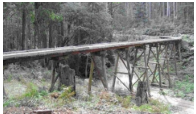
15000' Siphon trestle bridge, named because of its distance in feet from the beginning of the tramline at the top of the haulage, has recently been reconstructed to original specifications
