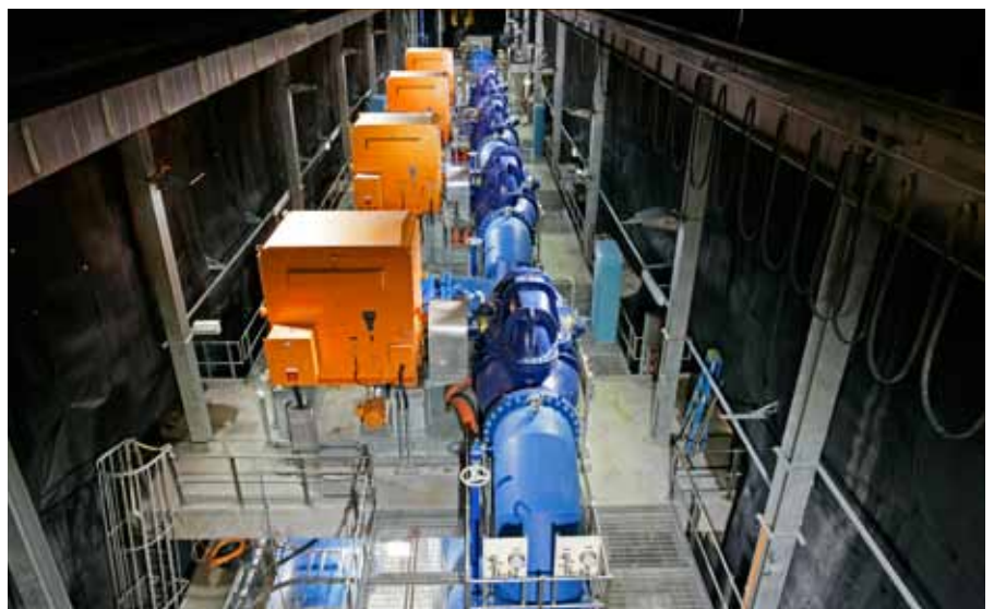
The new deep water pumping station at Warragamba Dam completed in early 2007, which, along with a deep water pumping station at Nepean Dam, provide access to previously inaccessible water, extending supply by around six months during drought.
