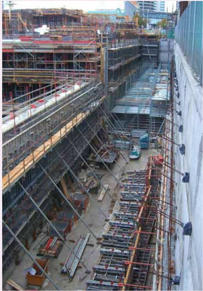
The detention tank under The Concourse at Chatswood can capture five million litres of stormwater.
