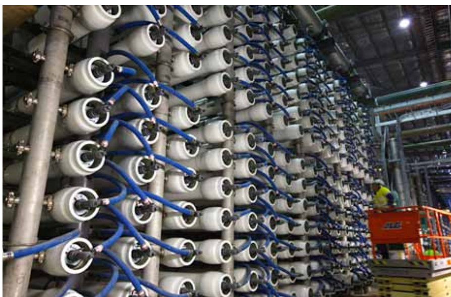
Reverse osmosis technology is used to extract salt from seawater during the desalination process.
