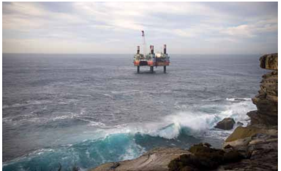
A jack-up barge, Seafox 6, was used as a drilling platform for the inlet and outlet shafts for the desalination plant. Construction of the plant was completed on time and under budget.
