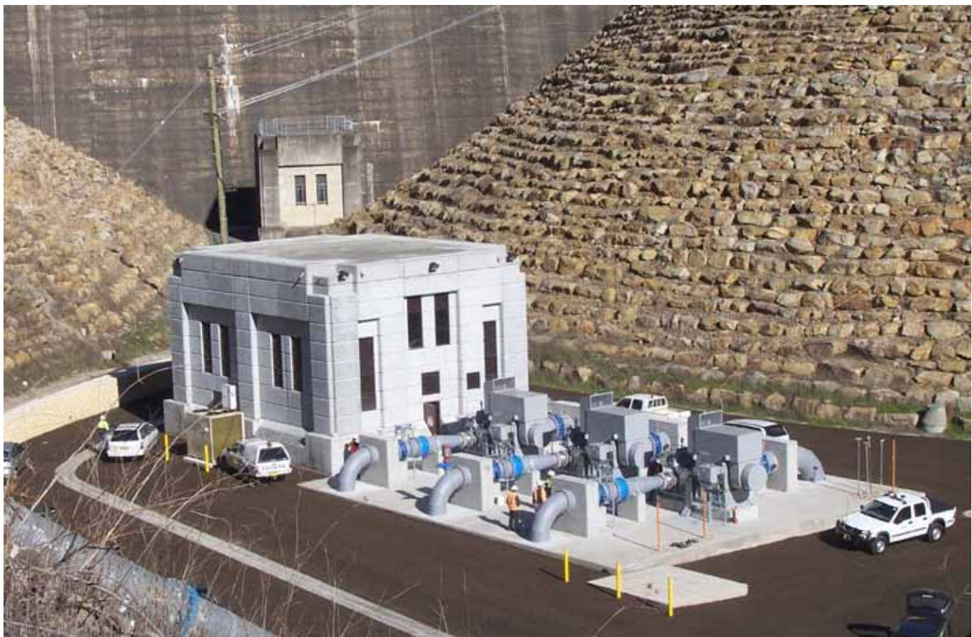
A new pumping station at Nepean Dam allows access to deep water and helps secure supplies to the Illawarra during drought.
