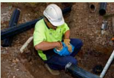
Sydney Water's leak reduction programs are estimated to be saving 30 billion litres each year.
