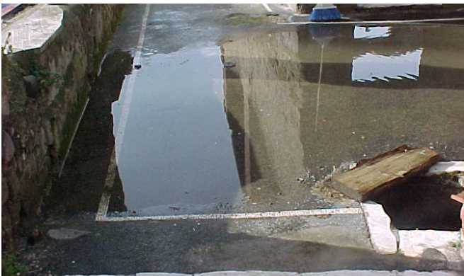
An example of the presence of water on site where the drainage system is not functioning. Note the drain in the bottom right hand corner which no longer adequately removes water due to changes in the slope of floor surfaces
