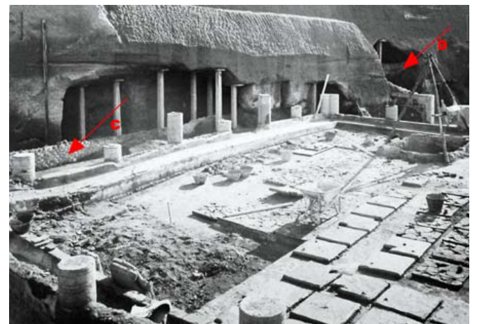
Photograph of the peristyle of the House of the Telephus Relief (Ins. Or. I. 2-3) during work to repair the tiled floor in 1937 (SAP Archive n° C 2746)
