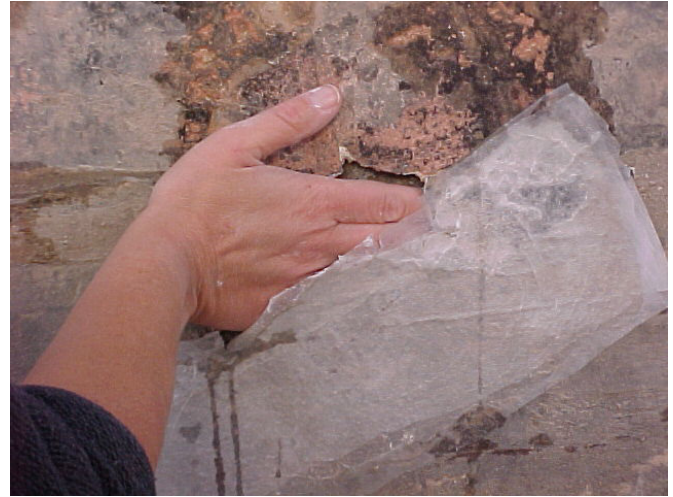
Detail of the detachment of preparatory layers of a wall painting from the supporting wall. The seriousness of this type of detachment is not particularly visible from outside, the surface (here protected by a provisional surface coating of Japanese paper) appears solid but the internal layers have disintegrated and are often completely missing
