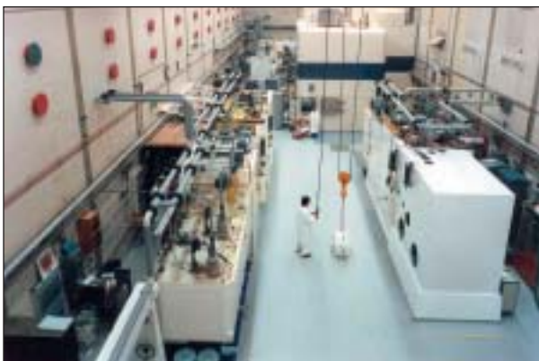
An interior view of the hot zone in the LHMA building today
