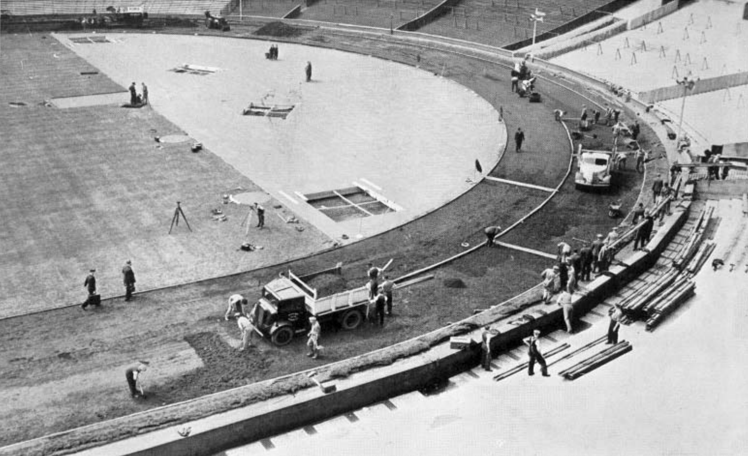
A general view of the work of laying the special track for the athletic events of the Games at the Empire Stadium, Wembley.
