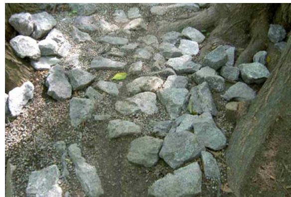
Trail in hardwood bush (FOD5-2), showing attempts to protect compacted tree roots and harden the tread with a layer of cobble-sized limestone, and gravel. Roots are protected from further damage by trail users, but may be susceptible to abrasion by the angular cobbles.
