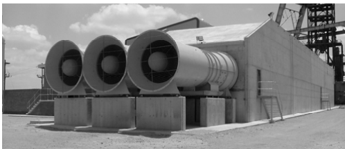
Figure 6. Air cooler fans of typical spray chamber.
