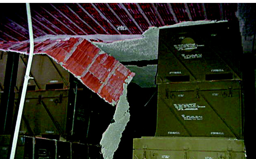
A portion of the collapsed ceiling in a munitions storage structure at Camp Darby, Italy. (Photos courtesy 31st CES)
