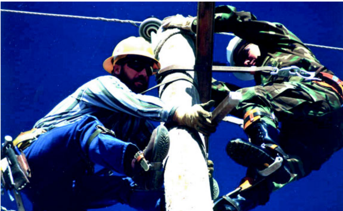
Dave King, Colorado Springs Utilities head training coordinator, trains A1C Adam Johnson, 21st CES, Peterson AFB, Colo., at the "pole farm." (Photos by Rob Bussard)
