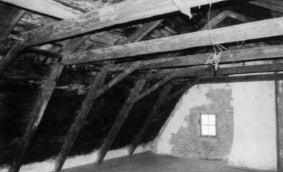
The loft of the Conyn/Van Rensselaer House Claverack, Columbia County, Photo by John Stevens, June 1999.
