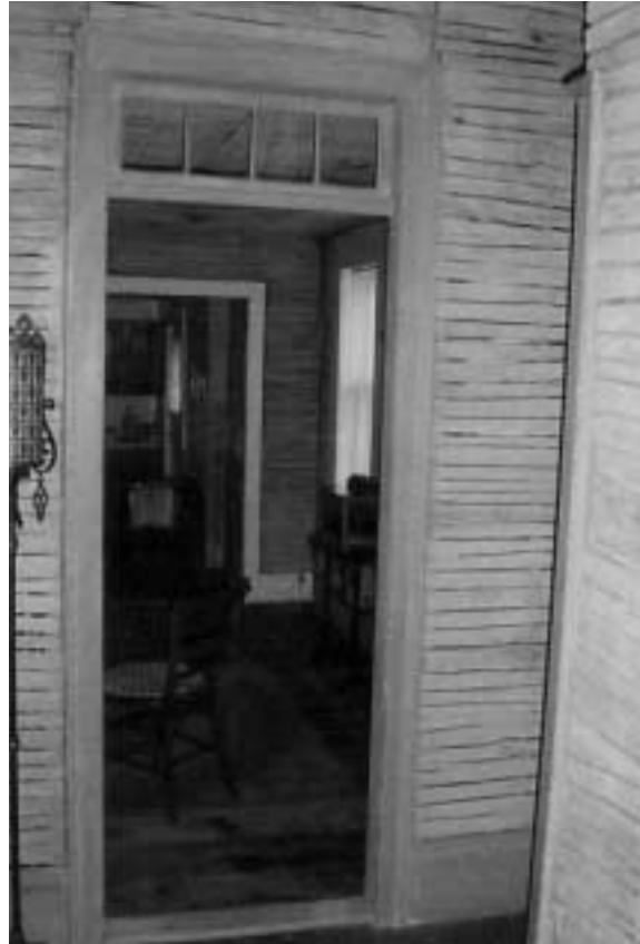
Dining room door from entry hall with original glass transom and handsplit lathing.
