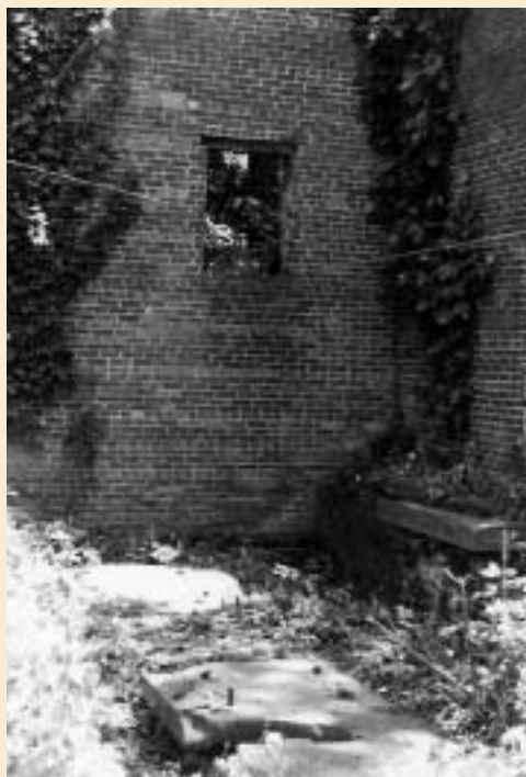
East view of the interior of the Nutten Hook Power House with window facing Ice House.
