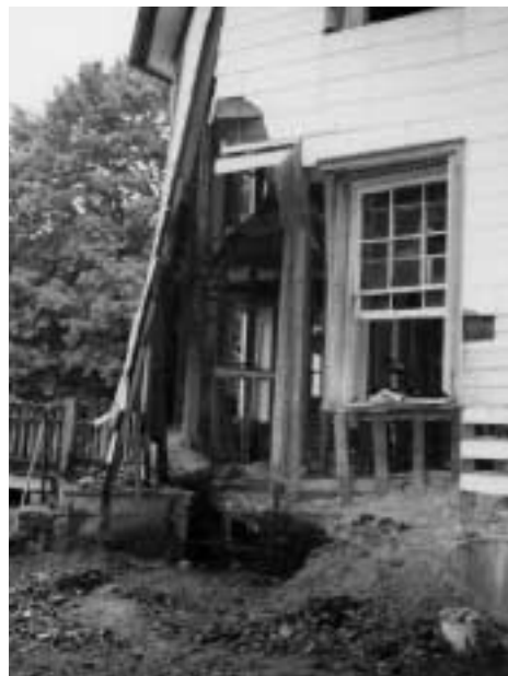
The abandoned house was badly treated by vandals and weather. Here the northeast wall is shown in partial collapse before restoration began.
