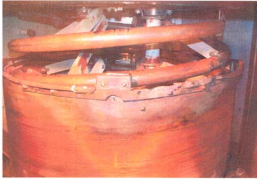
Figure 4: Worn and patched shorting drum (inside of transmitter) at site A.
