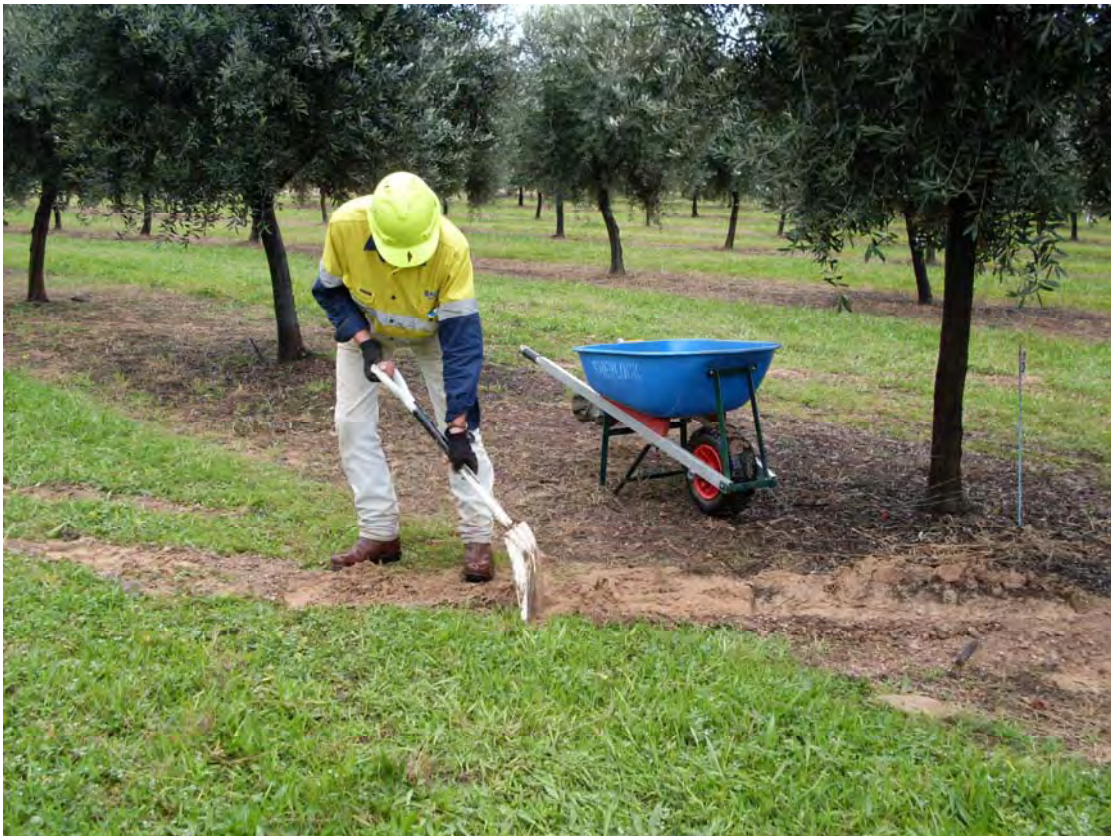
Plate 2-5 Subsidence repairs using wheelbarrow and shovel in the 'Atulya' olive grove over Longwall 11
