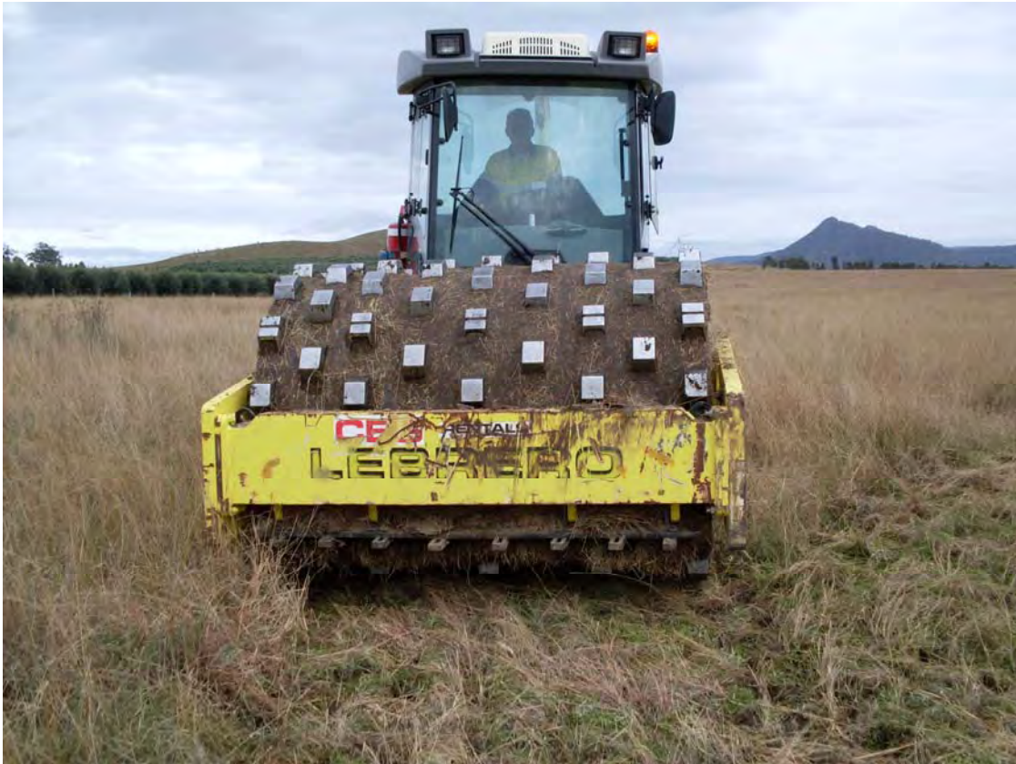
Plate 2-6 Subsidence repairs using a vibrating sheeps foot roller in open grassland above Longwall 11
