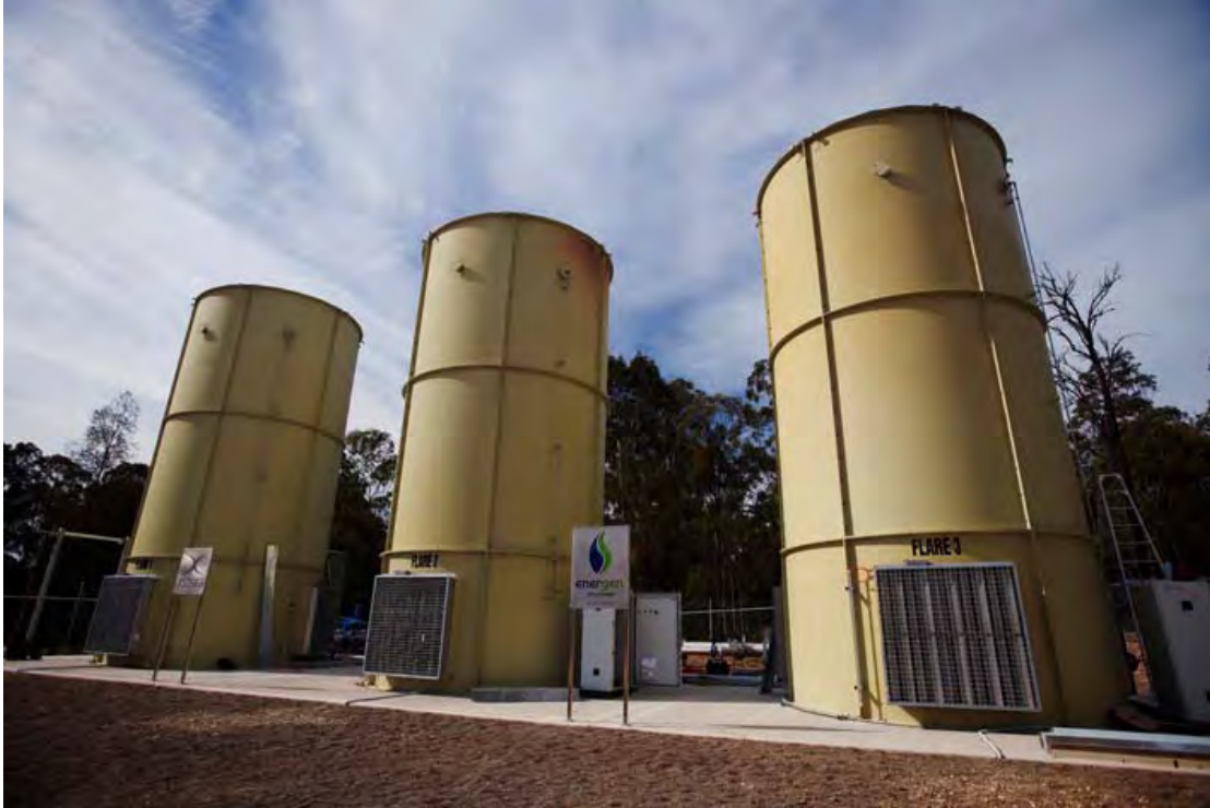
Plate 2-2 The new Energen methane flaring facility installed at the Underground Operations during 2009
