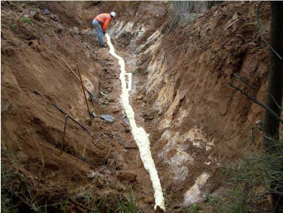
Plate 2-7 Polyurethane resin being used to seal cracking in sandstone along the Northern Drainage Line
