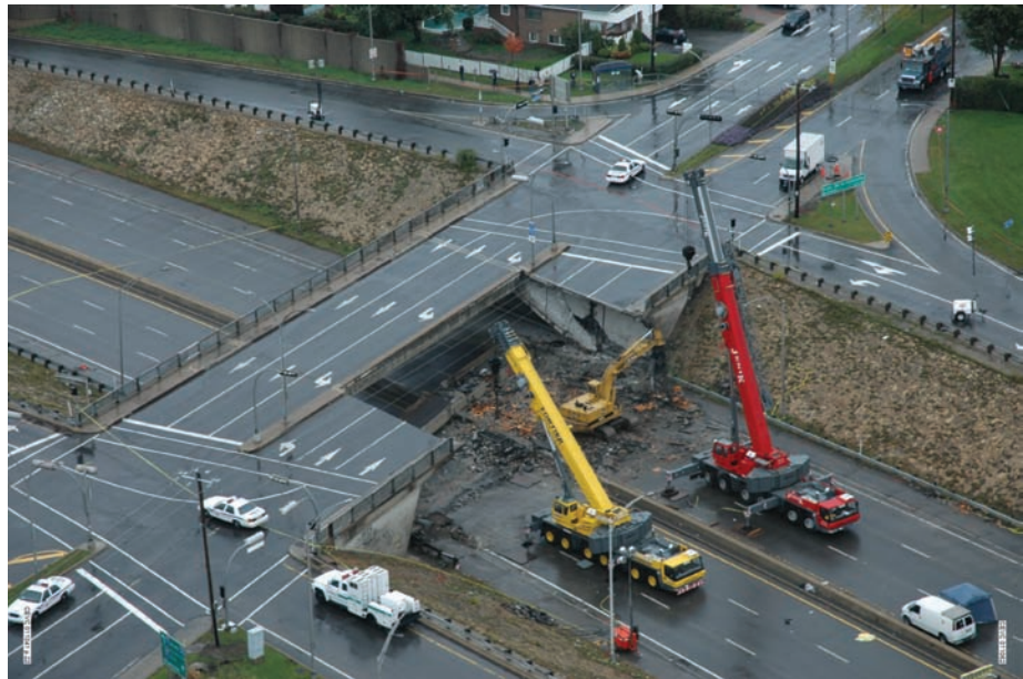
Figure 3.1 Collapsed Portion of the de la Concorde Overpass 3
