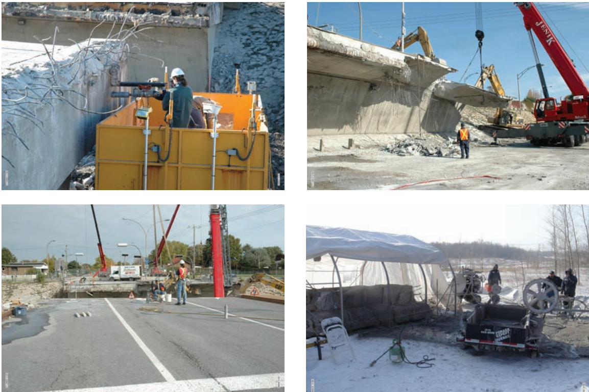
Figure 5.1 Operations carried out on the site of the collapse and on the Belgrand Street storage site
