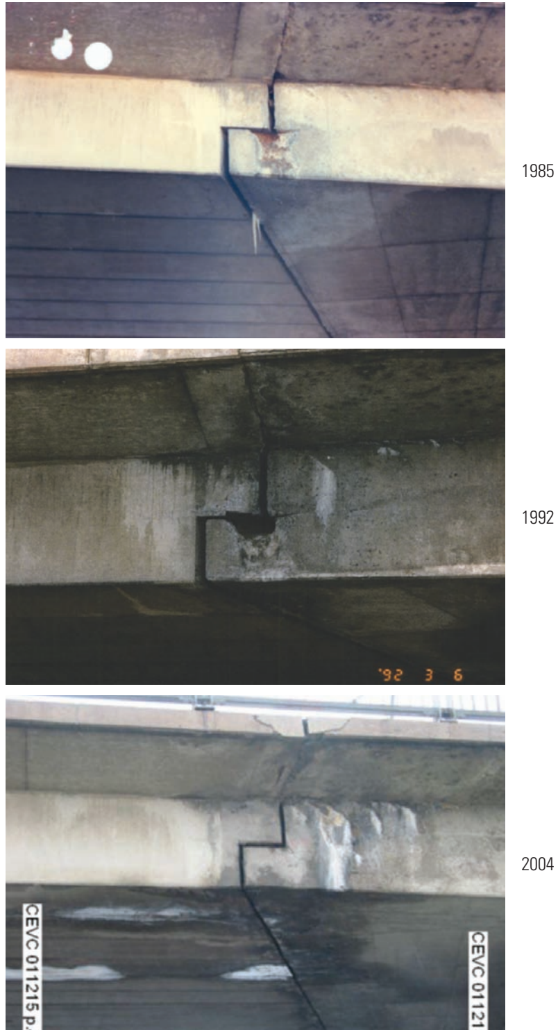
Figure 5.6 Views of the east cantilever, from the south side of the de la Concorde overpass, showing the evolution of cracks in the bearing support area 78
