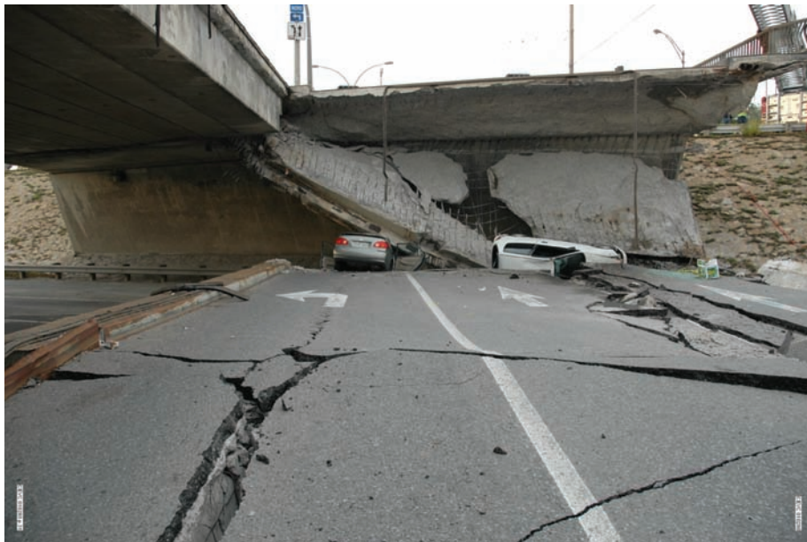
Figure 6.2 Front view of the east abutment shortly after the collapse, on September 30, 2006 2
