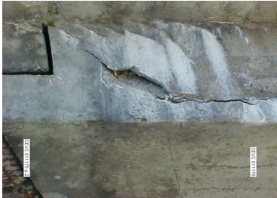
Figure 3.3 Hole and Crack in the East Abutment, photographed by Mr. Bonin between 11:45 a.m. and 12:00 p.m., September 30, 2006.
