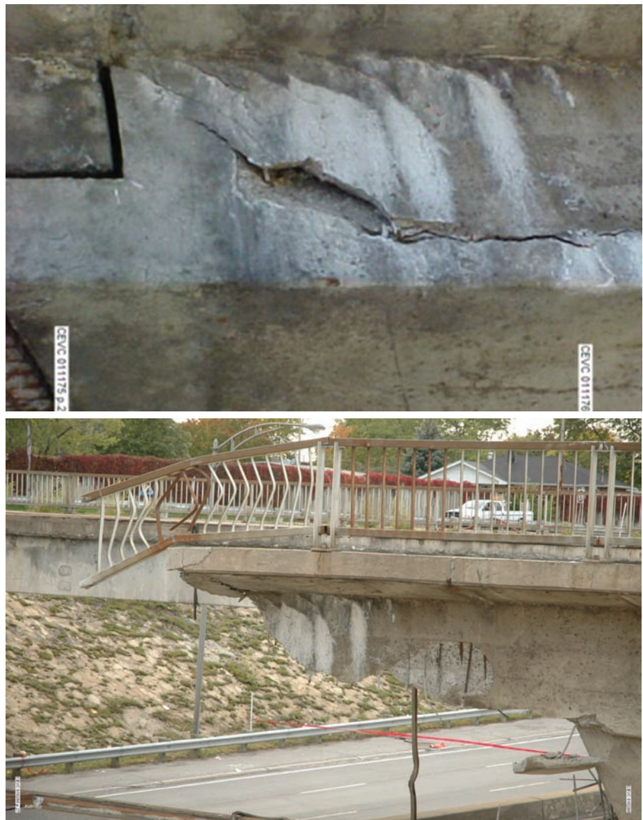
Figure 6.1 Vertical face of the south side of the east abutment, near the corbel: a) Top: picture taken by Jules Bonin on September 30, 2006, less than 60 minutes before the collapse b) Bottom: after the collapse
