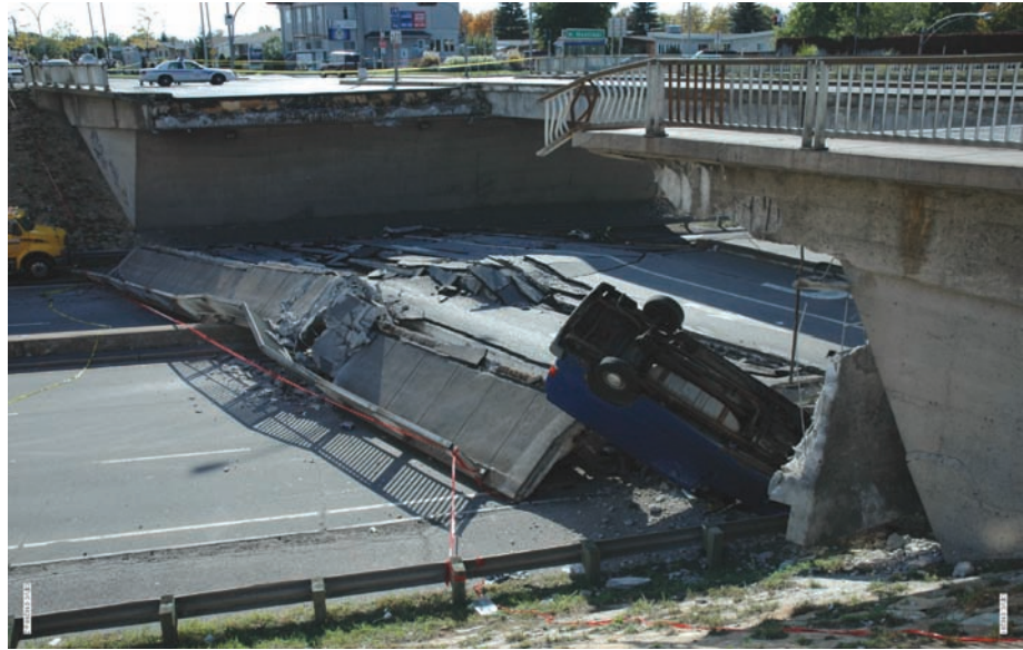
Figure 6.3 View looking to the west of the collapsed overpass, from the east abutment, on September 30, 2006 3
