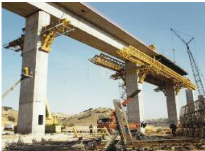
Underslung traveller for span-by-span construction process (movable shuttering system), Anchuelo viaduct high-speed railway Madrid-Barcelona (Spain).
