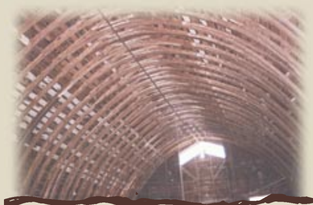
Wood was soaked in the farm pond so it could be bent to shape of roof— Holmgren farm dairy, Tremonton, Utah
