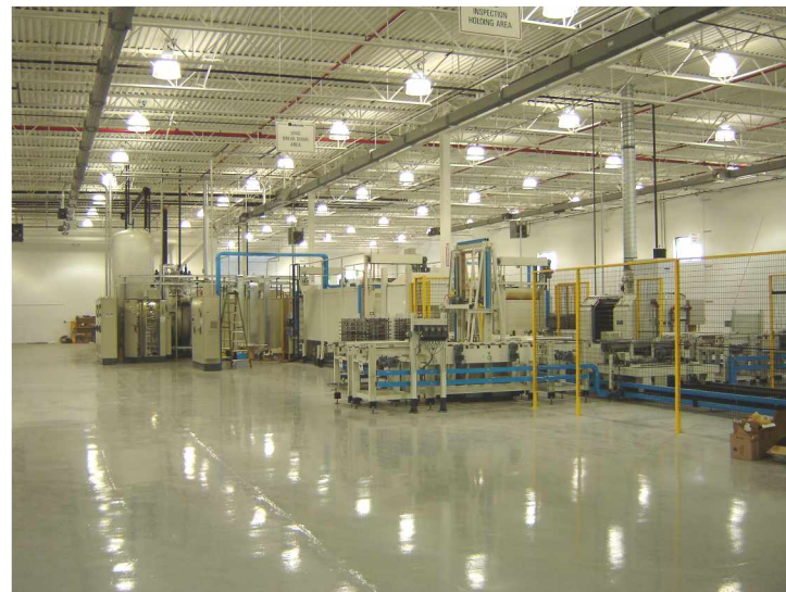
Fully automated handling equipment moves parts through cleaning, preheating, carburizing, quenching and tempering operations in the cell
