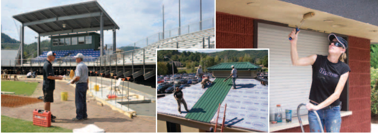
From left, Moranda works with Mackie McKay, a contractor who helped design parts of the project. Renovations included new roofing throughout the baseball stadium. Pamela Moranda, Coach Moranda's wife, puts some finishing touches on the stadium.
