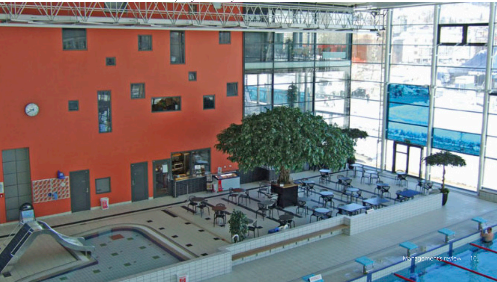
Five DanX 12/24 pool ventilation units installed at Norway's largest swimming baths - Drammensbadet
