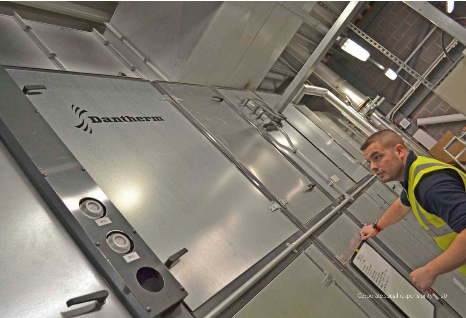
Service inspection of DanX 16/32 swimming pool unit at Spiceball Leisure Centre, Banbury, UK
