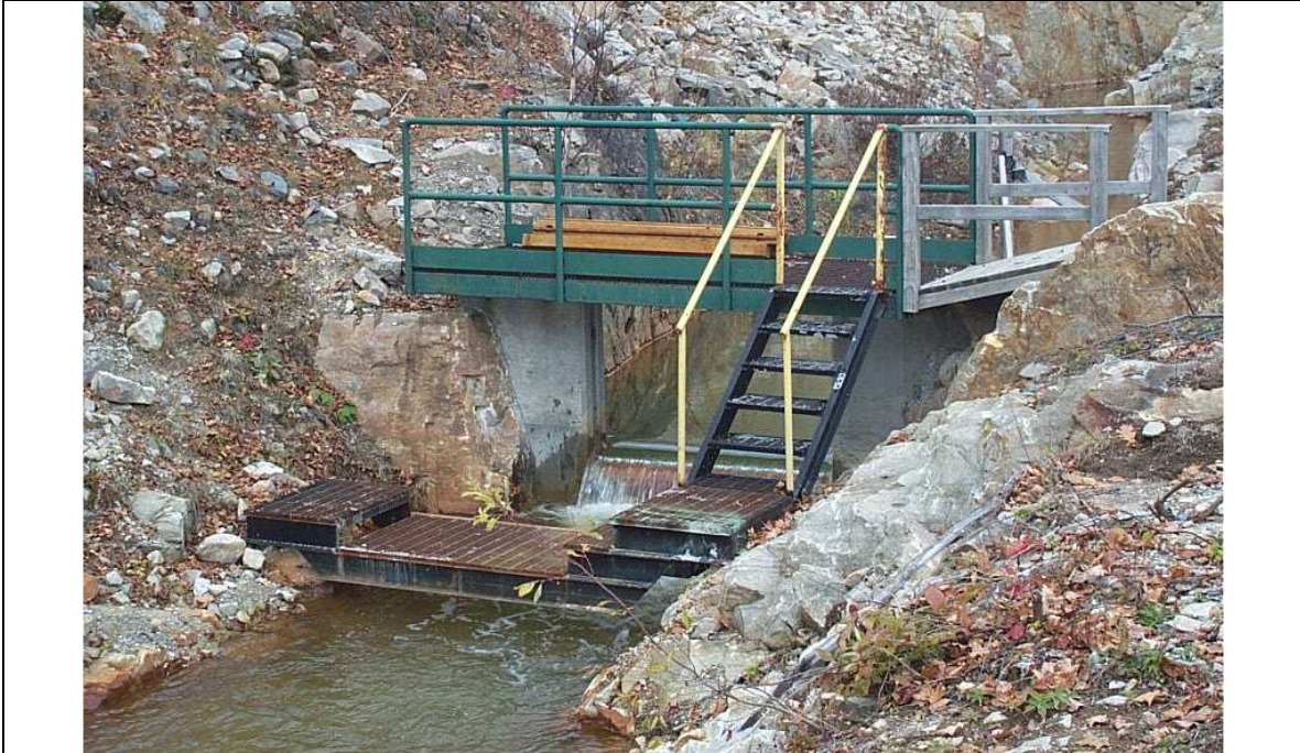
Photo 1: Nordic Settling Pond control structure
