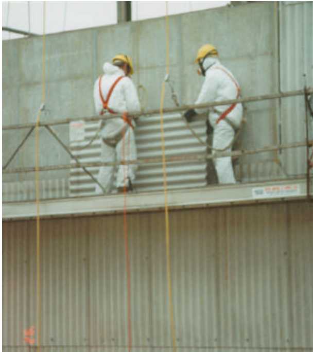
Asbestos siding removed by specialty contractor; disposal in dedicated asbestos landfill site in tailings management area.
