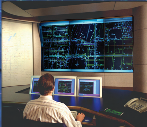
WorldView • Master Stations • SCADA Systems
