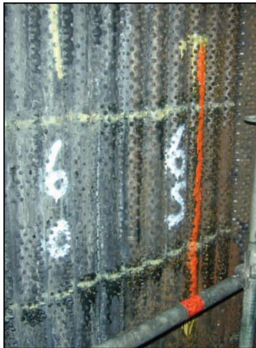
Figure 1. Lower furnace studded tubes can become thin and difficult to test with UT between the studs. Thinned tubes can be seen in the orange area.
