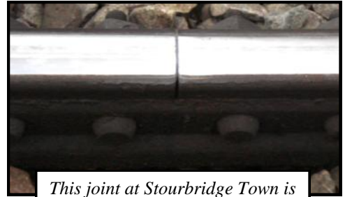
This joint at Stourbridge Town is so well made that the railcar passes over without noise or impact. Using lightweight vehicles, it will become easier to keep the track in this condition
