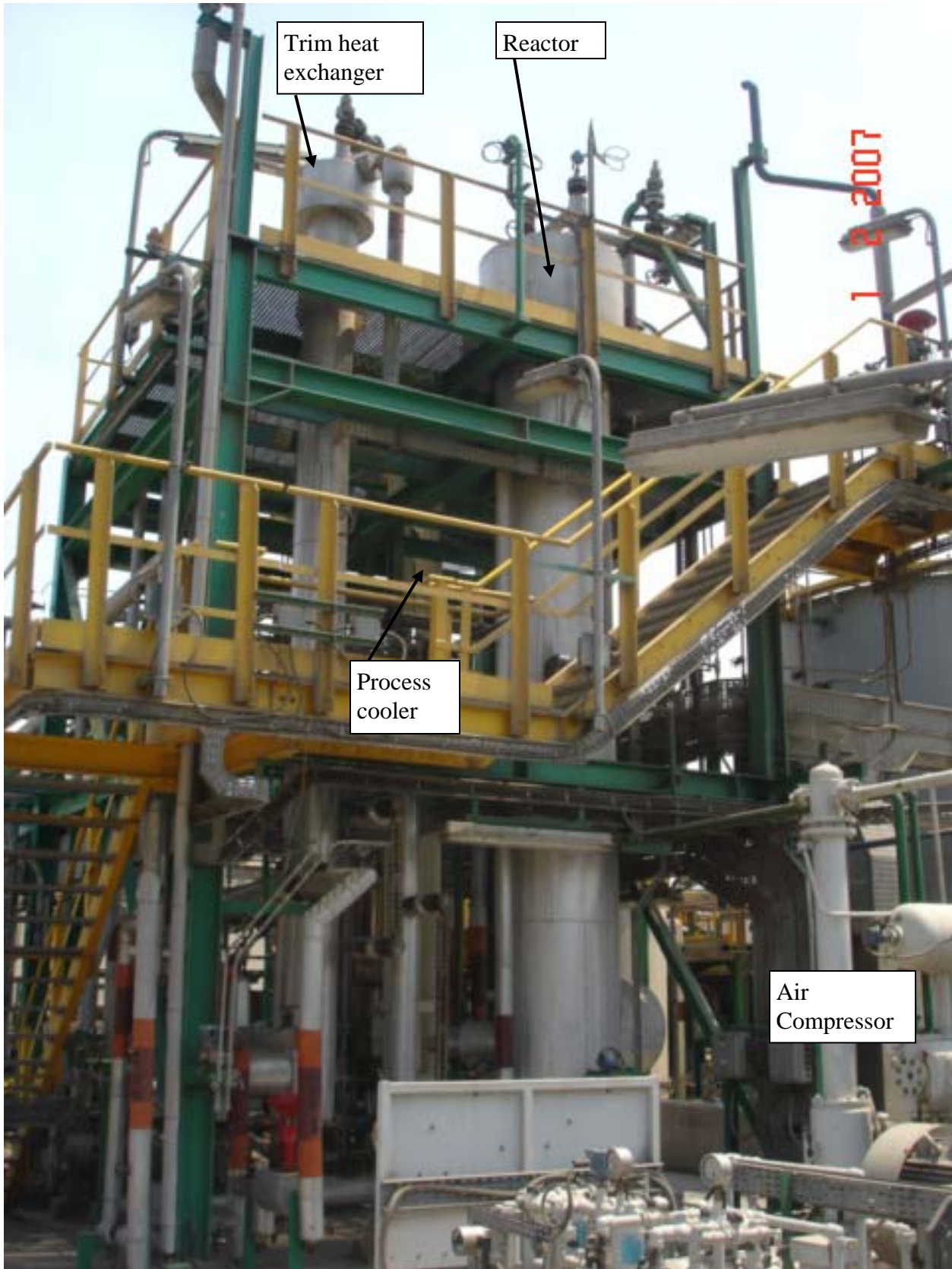
Figure 3. WAO system oxidation tower.
