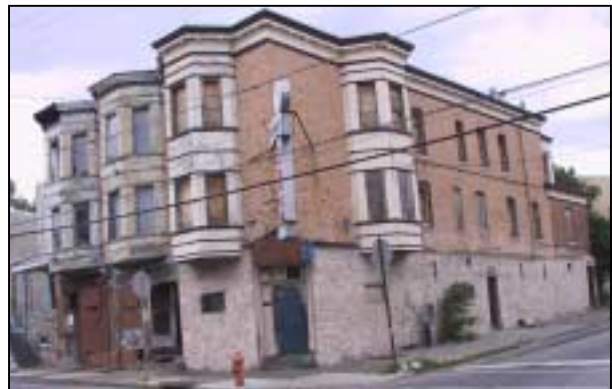
Blighted conditions: three vacant buildings on Wister St.
