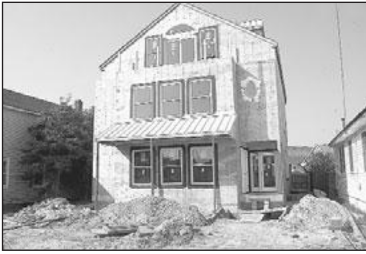
The Manasquan Planning Board agreed Tuesday night to allow applicant Michael Lynch to keep a 3-foot exterior wall, which violates borough zoning code, that he had constructed at a residence located at 557 East Main St.
