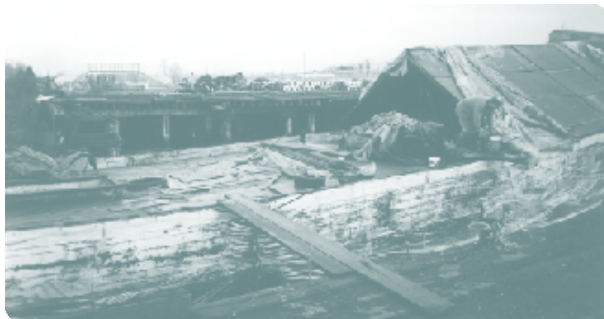
The plywood roof is used to keep rain water from flooding the hull
