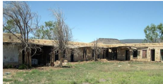
Photograph 20. Old motel, unique facade treatment; once lit up night sky with architectural neon.
