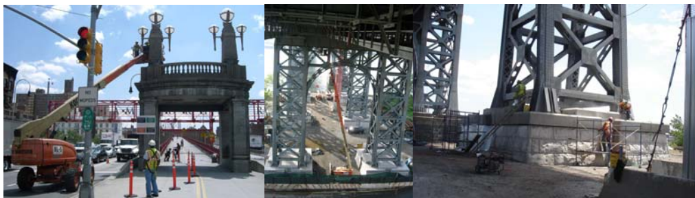
Contract #8 in 2008: Continuing the Installation of Luminaires at the Manhattan Plaza Bridge Entrance. New Bearing Replacement Preparatory Work. New Granite Cladding at Pier 15W.
