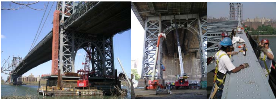
Contract #8 in 2004: Pier Stationed & Barge Mounted Cranes at Brooklyn Main Tower Pier. Steel Arch Replacement. Looking West at the North Truss Top Chord Steel Rehabilitation.
