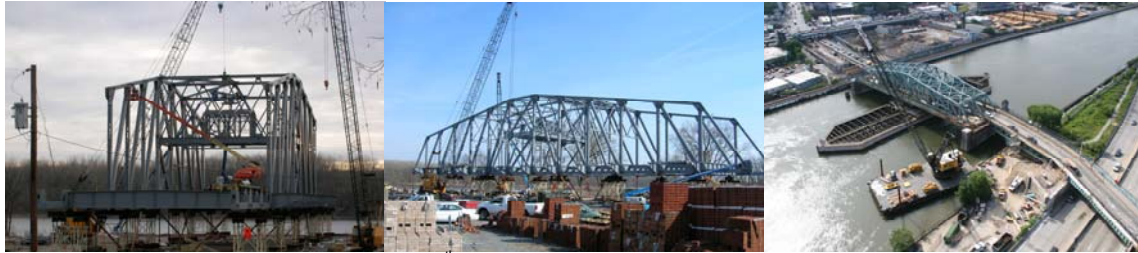
2006: Continued Assembly of the New 145 th Street Bridge Swing Span. Removing Steel Girders Over the Harlem River Drive.
