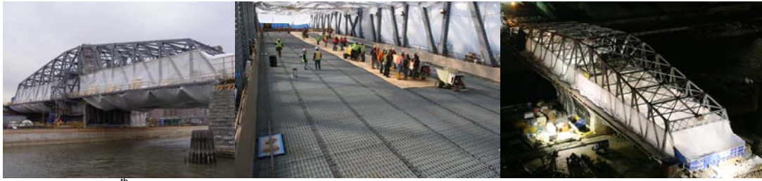
2007: New 145 th Street Bridge Swing Span Wrapped in Plastic During the Lightweight Concrete Curing Period. Preparing for the Concrete Deck Placement. Night View of the Encapsulated Deck.
