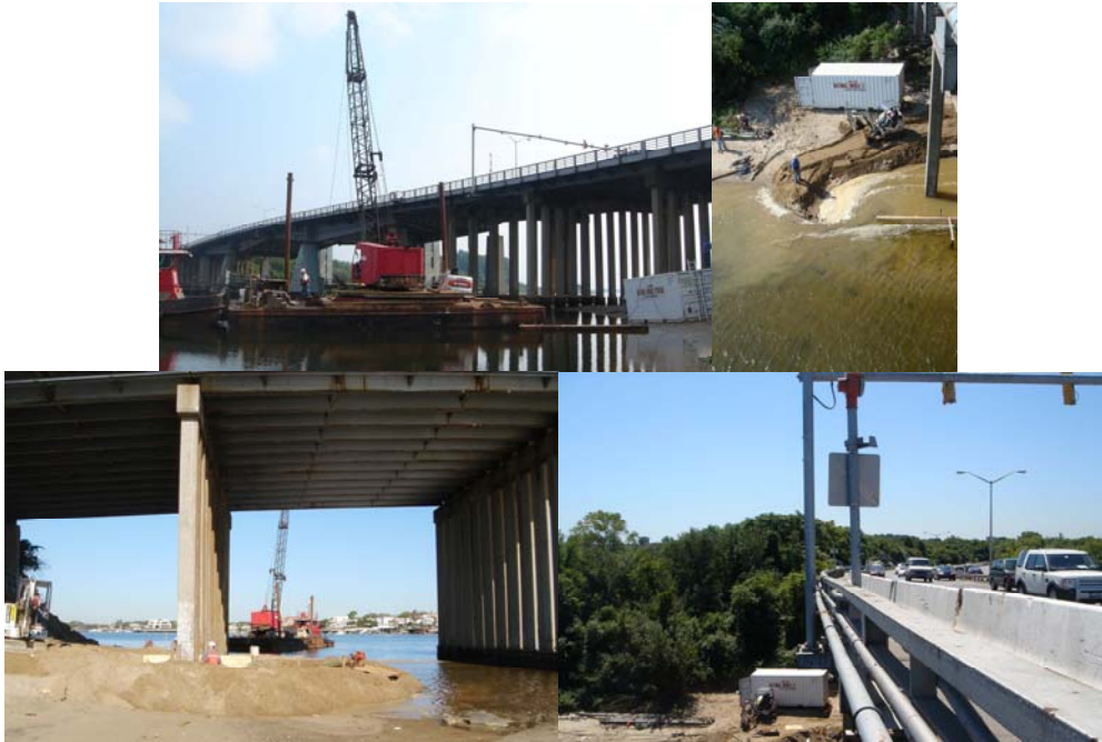
Mobilizing the Barge and Container. Installing the Barrier Wall Around Columns 13 and 14. The Barrier Wall System at Low Tide. General View of Belt Parkway over the Work Area Below. (Credit: Thomas Leung)
