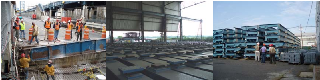
Contract #11 in 2006: Removal of First Floorbeam for Lower Roadway Reconstruction. The Fabricated Steel, Complete With Bearings, In The Contractor's Storage Yard.
