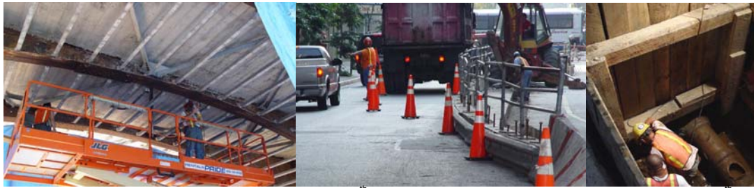
Contract #6 in 2004: Repairing the Steel of the 59 th Street Arch Ceiling. Starting Curb Replacement at 60 th Street. Improving the Drains at the Vehicle Storage Area.
