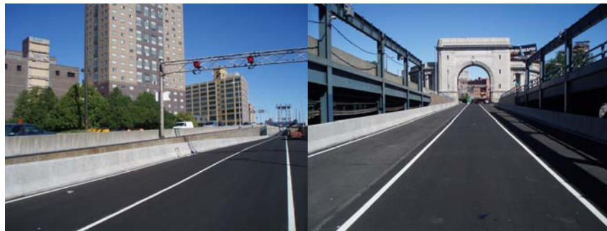
Contract #11 in 2007: The Completed Lower Roadway on the Brooklyn Side And Near the Manhattan Colonnade.
