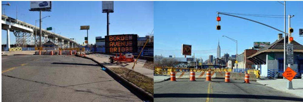
Borden Avenue Bridge Closed for Emergency Repairs. (Credit: Bernard Ente)
