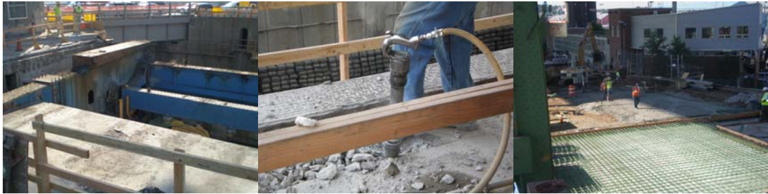
Removing the Existing Hamilton Avenue West Bridge Structural Steel in June 2008. Removing the Existing Southwest Toe Joint and Installing New Reinforcement of the Southwest Approach Slab in July 2008.
