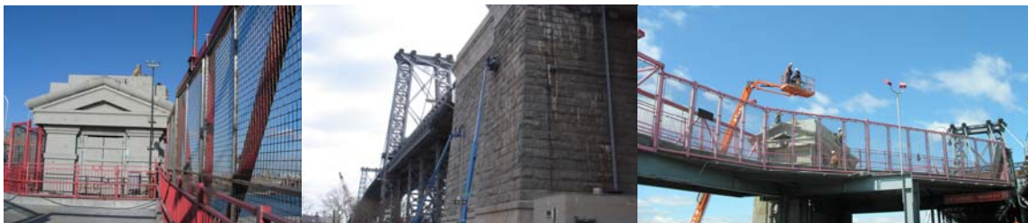
Contract #8 in 2006: North Comfort Station. Manhattan Anchorage Joint Cleaning and Painting. Pointing of Comfort Station Roof.
