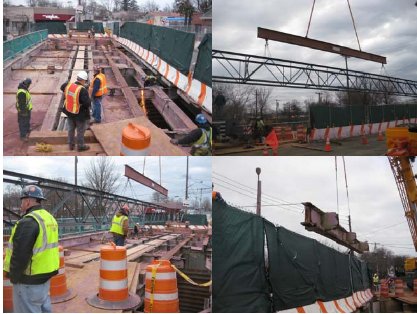
Annadale Road: Stage I Construction. Saw Cutting the Diaphragms, Removing the Stringers, And Placing a Temporary Truss to Support Utility Conduits.
