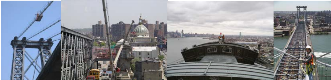
Contract #8 in 2005: Cable Band Bolt Retensioning. (Credit: Bojidar Yanev) Demolition of the Brooklyn South Comfort Station Balcony. Installing Brooklyn Main Tower Aviation Lights. FHWA Engineering Intern River Hwang Inspecting the Cable Wrapping.
