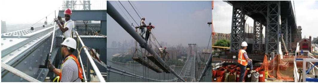
Contract #8 in 2004: High Strength Bolt Torque Inspection. Cable Band Bolt Retensioning. Steel Bracing Replacement Operation at the Brooklyn Intermediate Towers.
