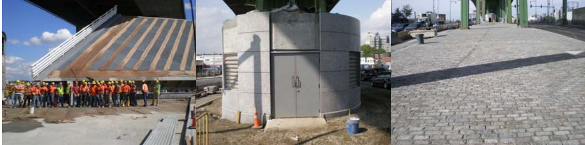
Completion of the New Hamilton Avenue West Bridge Installation in August 2008. Construction of the New Back Up Generator Building in September 2008. New Granite Pavers at the South Median Area in October 2008.
