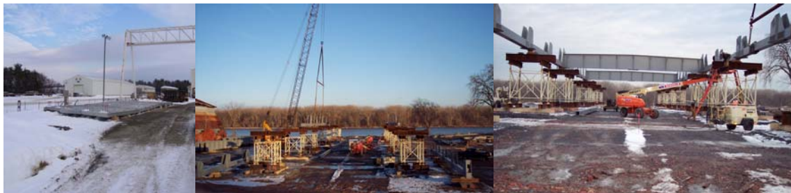
2005: Precast Deck Units for the 145 th Street Bridge at the Fabrication Facility. Placing the Bottom Chord of the Swing Span on the Supporting Towers.
