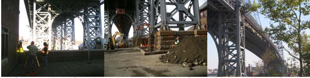
Contract #8 in 2007: Survey Work in Brooklyn. Excavation for Concrete Encasement. Brooklyn Tower.
