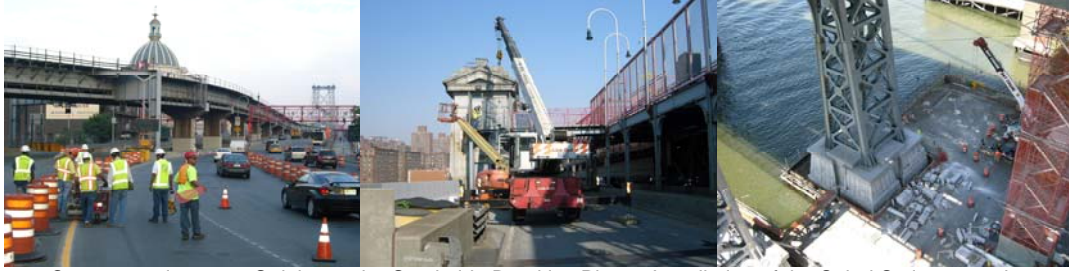
Contract #8 in 2008: Striping at the Southside Brooklyn Plaza. Installation of the Spiral Staircase at the Manhattan South Comfort Station. New Granite Cladding at Pier 20E.
