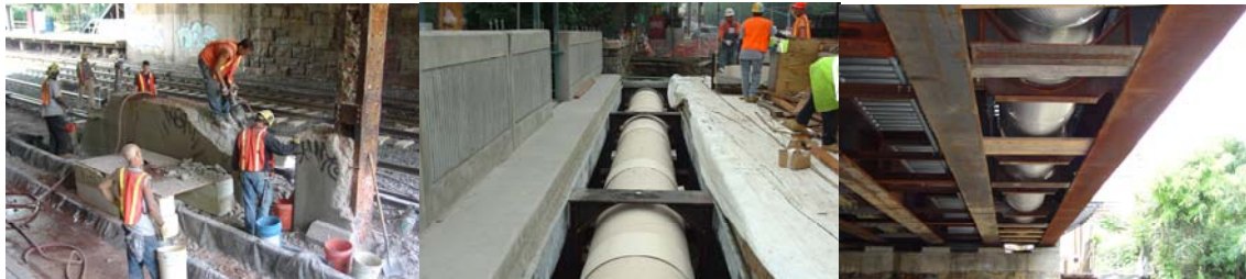
Gun Hill Road Bridge in June 2007: Looking Southwest at Laborers Demolishing the Existing Center Pier. July and August 2007: Installing a New Water Main.
