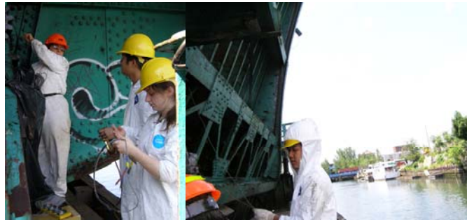
Assistant Mechanical Engineer Vera Ovetskaya and Summer Interns Samantha Shropshire and Edward Yee Checking Measurements at the Union Street Bridge in June 2008. (Credit: Ibrahim Ibrahim)
