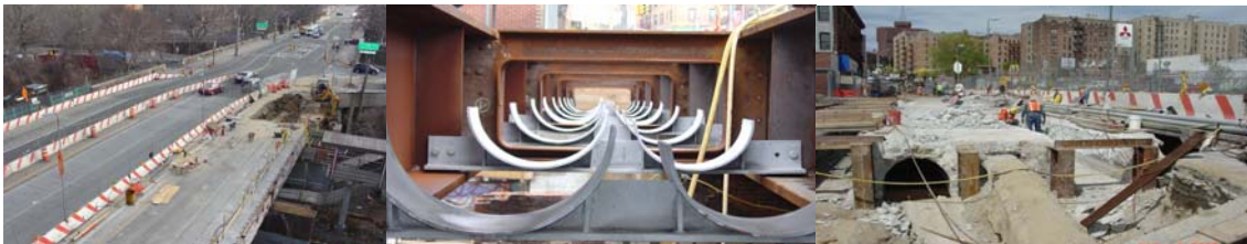
Gun Hill Road Bridge in January 2006: Stage 2 Construction Zone, South Side of Bridge. March 2006: Looking West From The East Abutment at The Utility Supports for The Gas mains. May 2006: Stage 2B Installing Shielding on Utility Bay.
