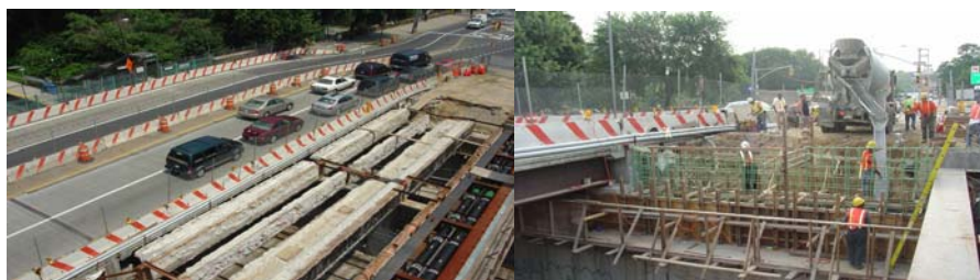
July 2006: Stage 2 Construction Zone, Prior to Girder Removal. July 2006: Looking East - Placing Concrete for The Gun Hill Road Bridge East Abutment Backwall, and a Quality Assurance Engineer Inspecting the Work.
