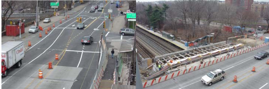
Gun Hill Road Bridge in December 2006: Looking East at the Stage III Traffic Shift, and Looking Northeast at Laborers Securing Plastic Covers on ECS Cables.
