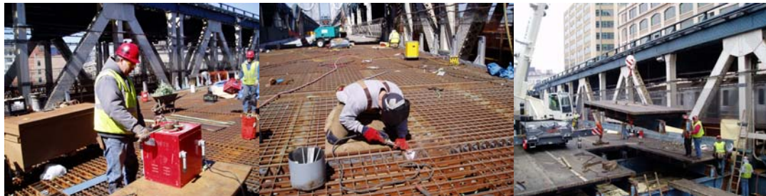
Contract #11 in 2007: Bending a Reinforcing Bar for the New Lower Roadway Grid Deck. Welding of the New Lower Roadway Grid Deck. Removal of the Existing Lower Roadway Grid Deck and Stringers on the Brooklyn Approach Span.
