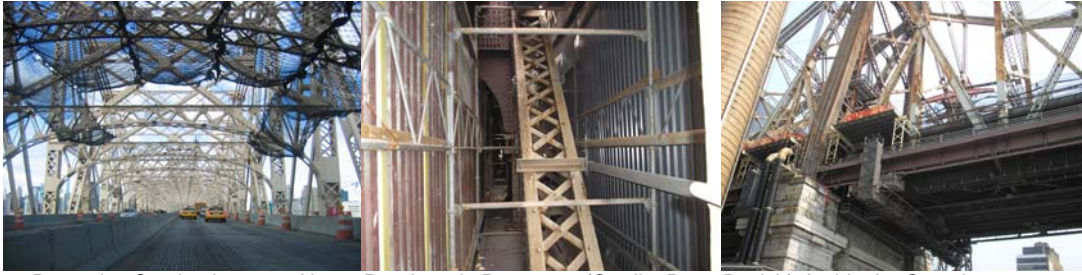
Protective Coating in 2006: Upper Roadway in Progress. (Credit: Peter Basich) Inside the Containment on the North Side of the Inner Roadway. Installed Platform Above South Outer Roadway.
