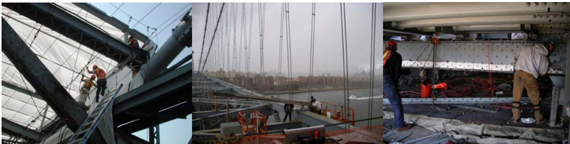
Contract #8 in 2003: North Stiffening Truss Containment Erection and Removal. South Truss Bottom Chord Rehabilitation.
