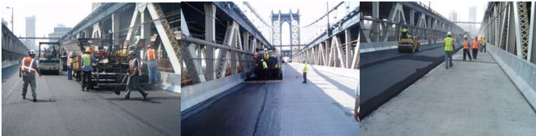
Contract #11 in 2007: Placement of New Asphalt on the Lower Roadway at the Brooklyn Approach Span. Placement of New Microsurfacing on the Lower Roadway at the Manhattan Side Span. Quality Assurance Engineers Yuliy Zak and Javed Sarwar Inspecting the Asphalt and Concrete on the Manhattan Approach of the Manhattan Bridge. (QA Credit: Masroor Mahmood)
