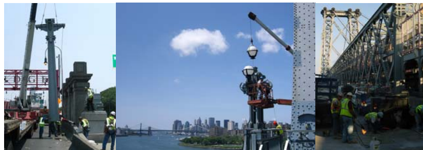
Contract #8 in 2008: Erection of the Manhattan Entry Electrolier. Installation of Electrolier Luminaires at the Brooklyn South Main Tower. South Outer Roadway Overlay Repairs.
