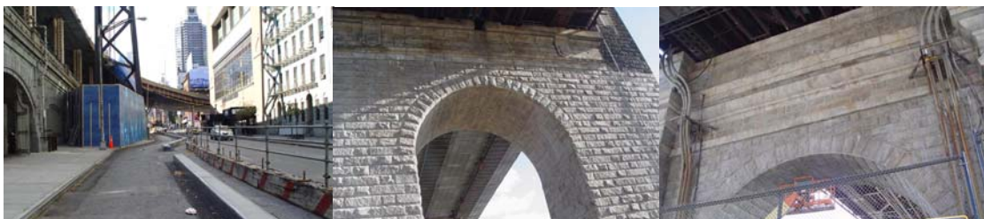
Contract #6 in 2004: Repaired Curb at 60 th Street. Anchor Pier Granite Cleaning in Progress.
