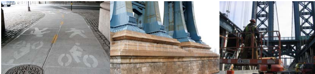
Contract #11 in 2008: Renovated Sands Street Bicycle Path in Brooklyn. New Railing at Base of Tower. Working on the Roadway. (Roadway Credit: Peter Basich)
