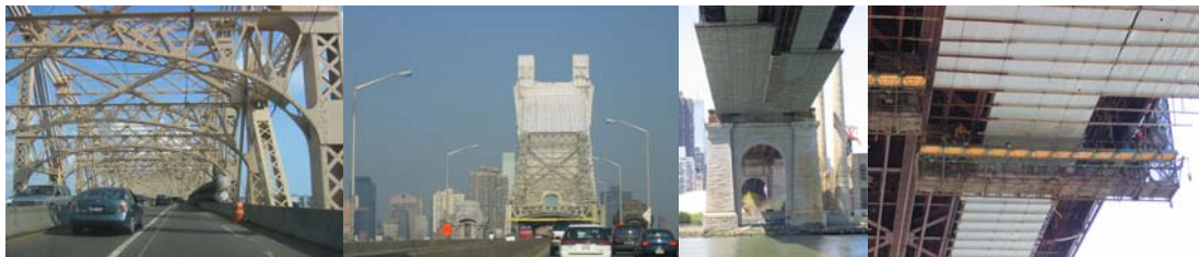
Protective Coating in 2005: Newly Painted Section Along the Upper Roadway. Containment on the Queens Side Tower. (Credit: Peter Basich) Queensboro Bridge Work Platform. Painters Arriving at the Platform. (Credit: Michele N. Vulcan)
