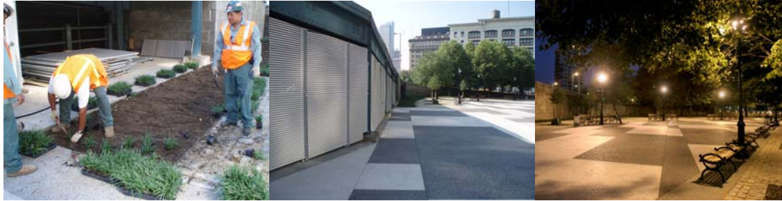
Installing New Plants. Completed Renovations. Evening View of the Plaza Looking Southeast With Benches, Lights, and Granite Pavers in Foreground.
