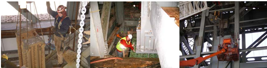
Contract #8 in 2005: Removing the Existing Steel of the Brooklyn Main Tower. Inspecting a Rebar Cage at the Manhattan Main Tower. Installing a Column at the Brooklyn Main Tower.
