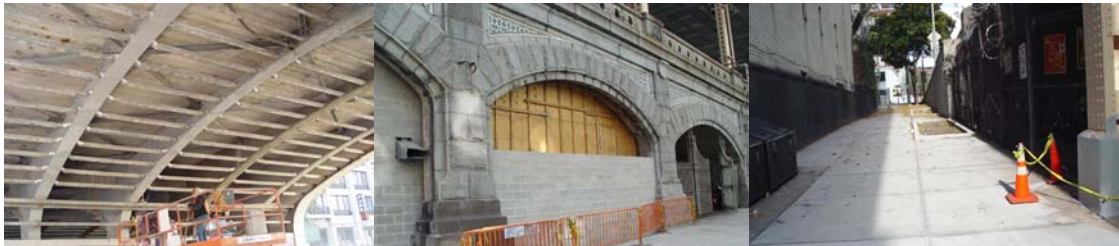
Contract #6 in 2004: Repairing Spalled Concrete at the 59 th Street Overpass. Sanitation Arch Infill Work Progressing at 60 th Street. Repaired Sidewalk Between 61 st & 62 nd Streets.
