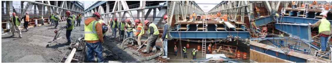
Contract #11 in 2007: Concrete Placement in the New Lower Roadway Grid Deck on the Main Span. New Lower Roadway Floorbeams, Stringers and Grid Deck on the Brooklyn Approach Span.
