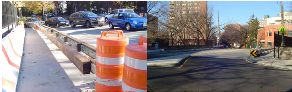
Newly Installed Steel-Backed Timber Guide Rail at West 239 th Street Bridge. Completed Bridge.
