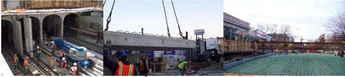
Installing Pier Walls for the 17 th Avenue Bridge. Installing Precast Deck Panels. Placing the Reinforced Concrete Bridge Deck.
