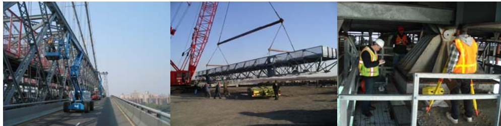
Contract #8 in 2006: Touchup Painting on the North Truss. First Traveler Platform. Bearing Survey.
