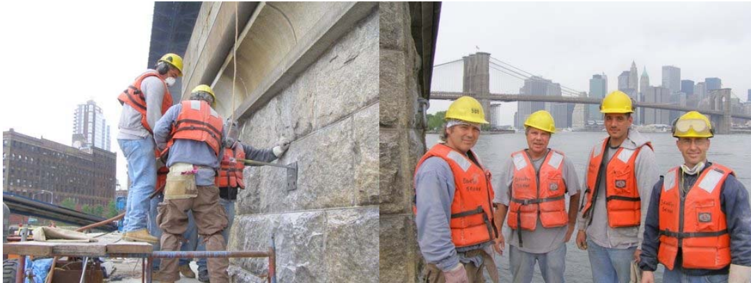
Cement Masons Installing Ladders and Mooring Rings for the FDNY on the Manhattan Bridge Towers. Cement Masons Victor Porowski, Paul Maguire, and Frank Finizio, and Bricklayer Vincent Sciulla. (Credit: Hany Soliman)
