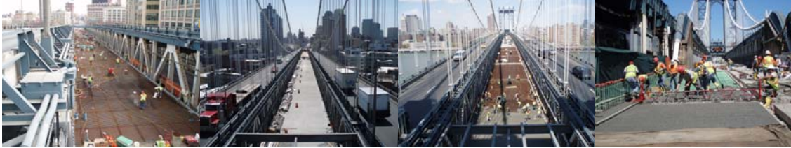
Contract #11 in 2007: The New Lower Roadway Grid Deck on the Brooklyn Approach Span. The New Lower Roadway on the Brooklyn Side Span After Concrete Placement. New Lower Roadway Concrete Placement on the Brooklyn Main Span, and at the Brooklyn Anchorage.
