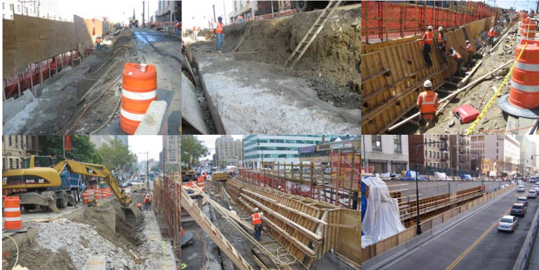
2007: Demolition and Reconstruction of the Northeast Retaining Wall of 161 st Street Between the Grand Concourse and Sheridan Avenue.
