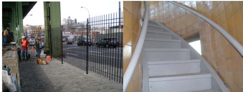
Installation of New Hamilton Avenue Parking Fence at the North Median Area in November 2008. Painting the Existing Control House Staircase in December 2008.
