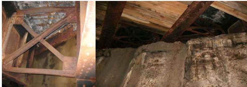
Deteriorated Bridge Deck With Exposed Rebar and Warped Steel Bracing Due to the Heat From the Fire. Timber Shielding on the Underside of the Bridge.
