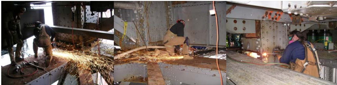
Contract #8 in 2005: Rehabilitation of the Brooklyn Main Tower Steel. Torch Cutting on the Tower.
