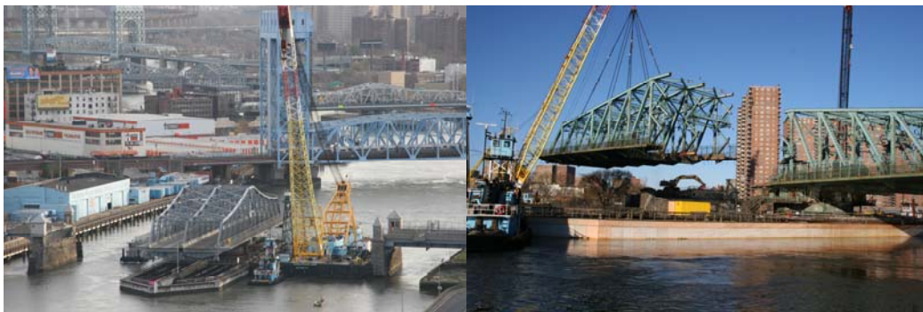
2006: Barge Carrying Crane Passing The Open Madison Avenue Bridge on the Way to Dismantle the Old 145 th Street Swing Span. Dismantling the Truss.
