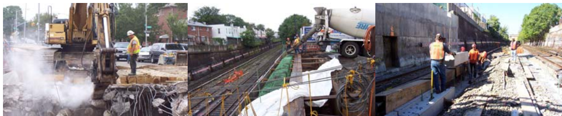
Demolition of the 17 th Avenue Bridge Deck. Casting the New East Abutment Wall. Installing Precast Concrete Footings.
