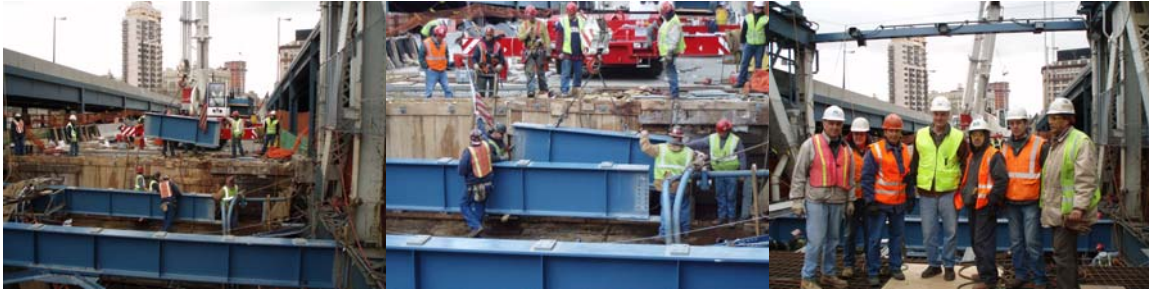
2007: Placing the Final Floorbeam Into Position. Engineer-In-Charge Brian Gill (in Center) and Inspection Staff on the Lower Roadway.
