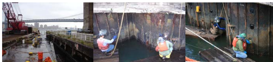
October 2007 - View of the Barge Equipment Blocking the East River Waves and Protecting the Crew Patching the Steel Wall. Dockbuilders Preparing Holes Prior to Welding Steel Patches on the Existing Cofferdam. Dockbuilders Applying Splash Zone Compound Over the Welded Steel Patch Plates. (Credit: Thomas Leung)
