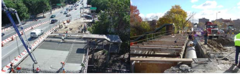
September 2006: Stage 2 Construction Zone, Placing Concrete for the Deck. November 2006: Looking East - Removing the Existing Water Main Pipe on the Bridge.
