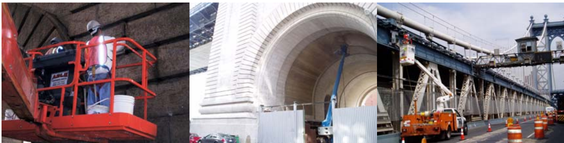
Contract #11 in 2006: Pointing Joints on East Face of Brooklyn Anchorage. Masonry Cleaning Inside Archway of Brooklyn Anchorage. Installing Conduit and Wire for New Lower Roadway Lighting.
