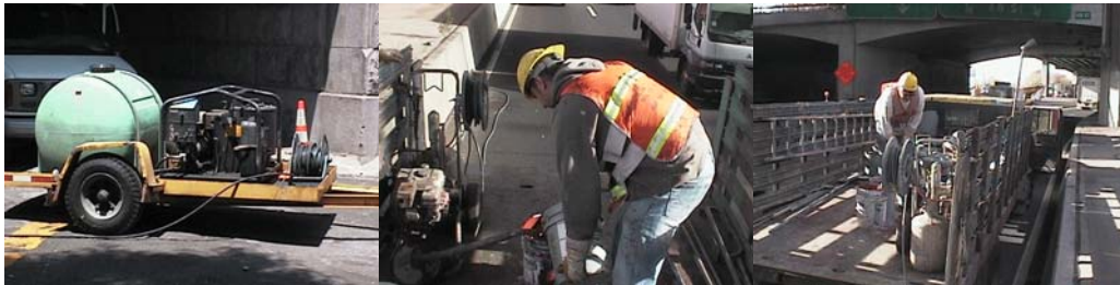
Pressure Washing Machine Used for Graffiti Removal. It is Set to 2500 psi and 212° F. Bridge Painters Frank Duic and Russell Newme Feeding the Spray Pump and Preparing the Paint.
