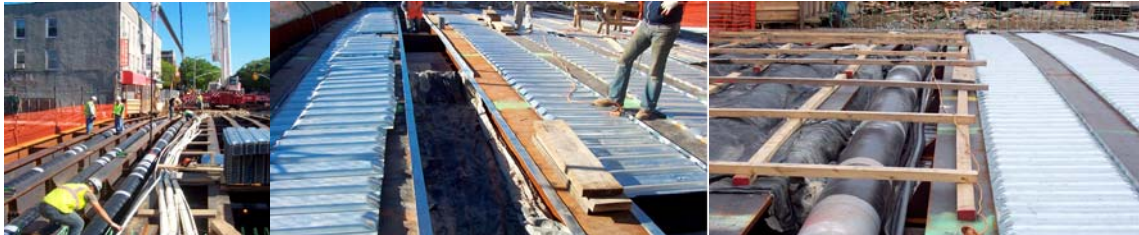
Installing the Gas Main Under the 20 th Avenue Bridge North Sidewalk in September 2007. Installing Metal Forms for the Bridge Deck in November 2007. Gas Mains Prior to Modification in December 2007.
