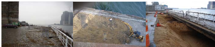
View of the Pavers Before Work Began to Stabilize the Area in December 2007. January 2008 - Top View of Backhoe Removing the Paving Blocks. Excavated Promenade Revealing the Exposed Steel Cofferdam Under the Concrete Walkway. (Credit: Thomas Leung)
