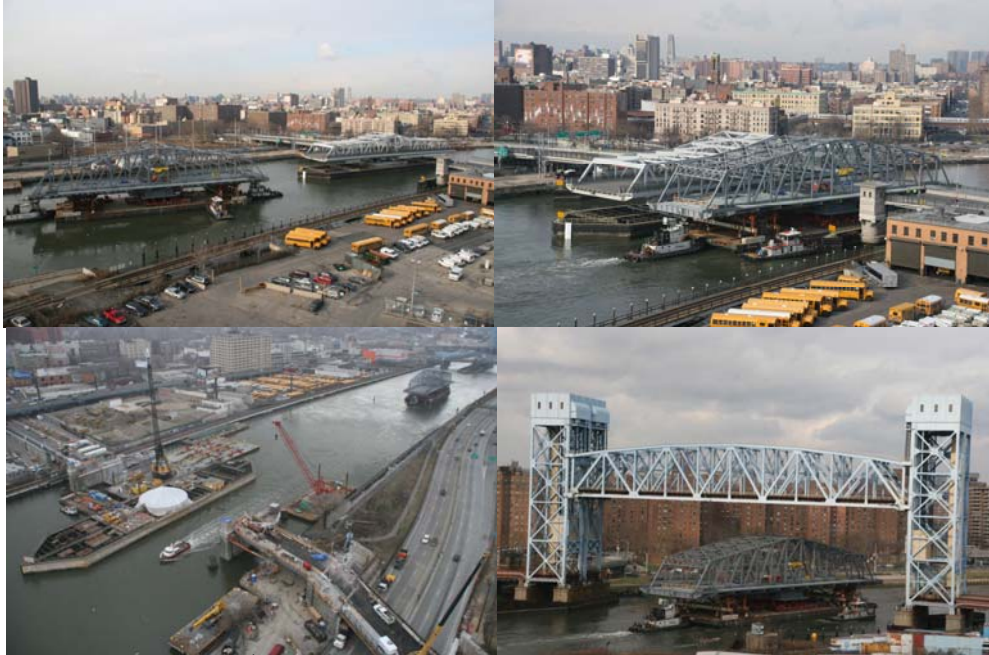
Moving the New 145 th Street Swing Span From South of the Third Avenue Bridge to the Site in January 2007. Passing Under a Metro-North Railroad Bridge.
