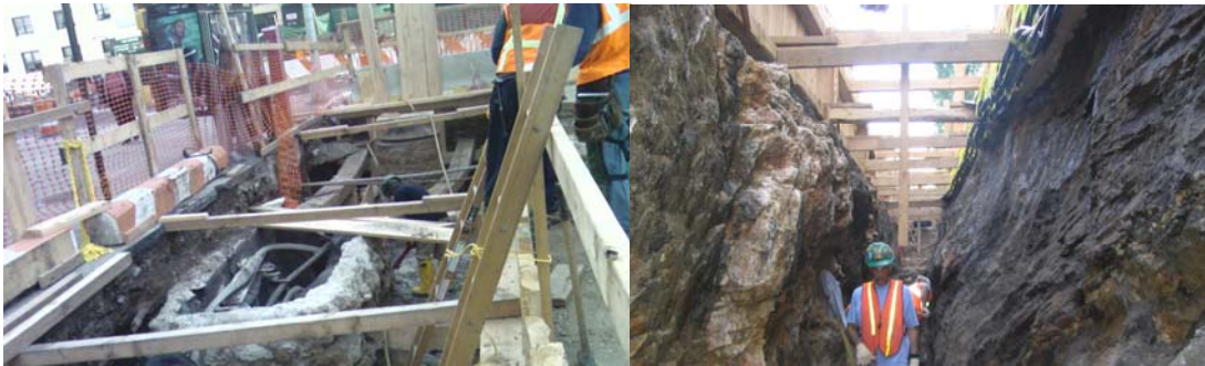
2006: Grand Concourse Bridge: Demolition of Existing Con Ed Vault. Backfill and Compaction of Sewer Manhole.
