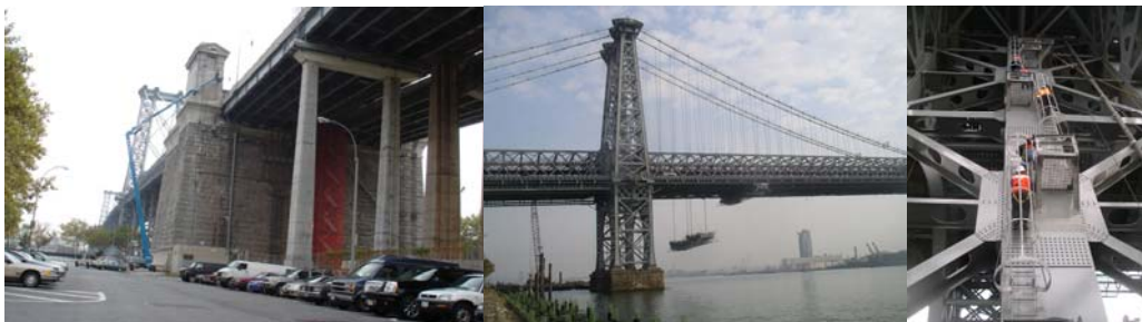
Contract #8 in 2007: Brooklyn South Comfort Station Rehabilitation. Raising the Manhattan Side Traveler at the Manhattan Tower. Manhattan Tower North.
