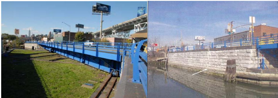
Borden Avenue Bridge. (Credit: Peter Basich) General View of the Crack in the Wingwall.
