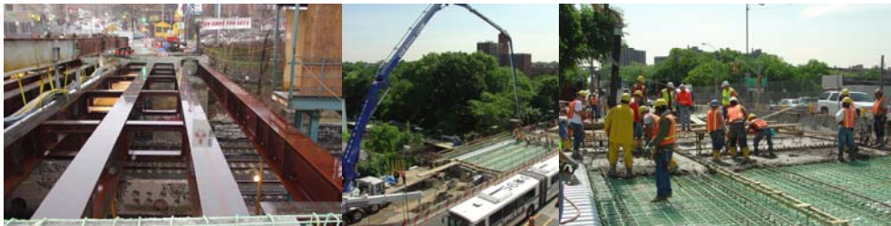
April 2007: Looking West – Gun Hill Road Bridge Stage III Girders and Temporary Support for Existing ECS Cables. June 2007: Using a Pump to Place Stage III Bridge Deck Concrete.
