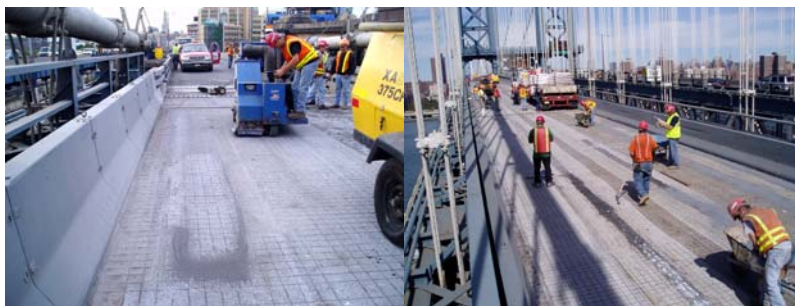
Contract #11 in 2005: Preparing the Deck for New Microsurfacing on the South Upper Roadway.
