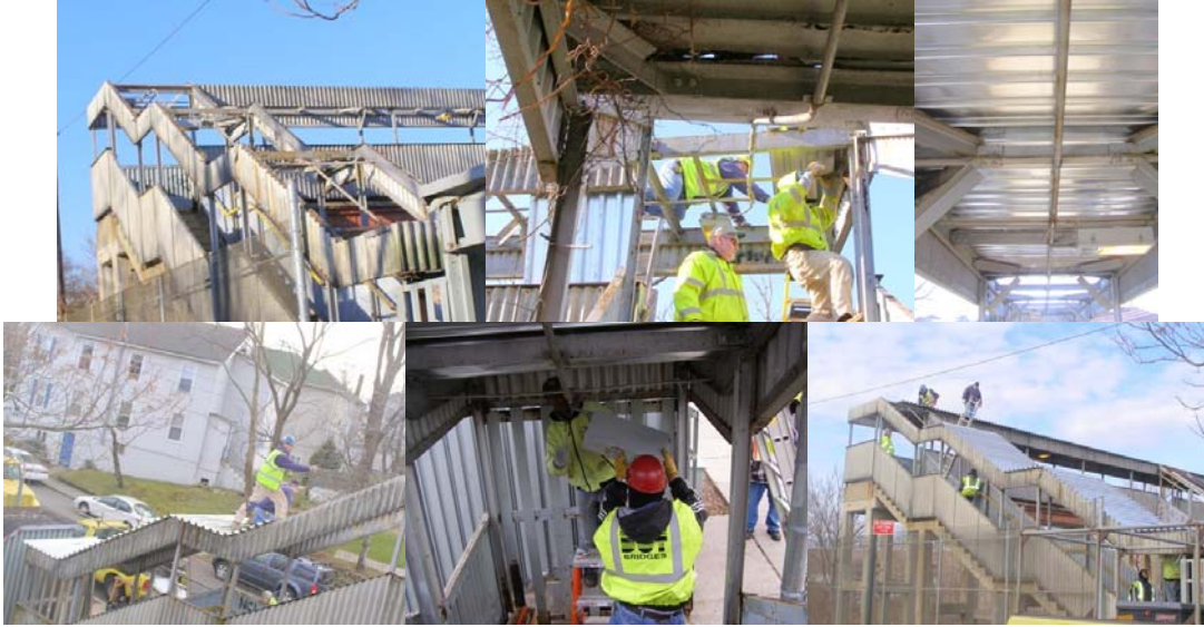
Carpenters and Electricians Replacing the Corrugated Roof and Lighting on the Bethel Avenue Pedestrian Bridge. Bridge View. Carpenter Michael Short III, Supervisor Carpenter John Motylewski, and Carpenter Mark Pavia. Roof Detail. Carpenter Pavia on the Roof. Electrician Gary Emmanuel and Supervisor Electrician Jose Done. Inspecting the Work: Carpenters Pavia and Short III, Supervisor Carpenter Motylewski, Carpenter John Green, and Electricians Emmanuel and Nelson Crooks. (Credit: Samuel Teaw)
