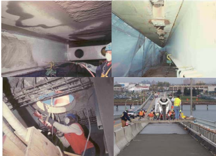
2006: Performing Underdeck Repairs. Working Inside the West Rebar Box Frame. Beam Repair. Concrete Placement.
