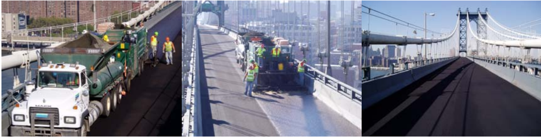
Contract #11 in 2005: Placing the New Microsurfacing on the South Upper Roadway. Newly Resurfaced Roadway.
