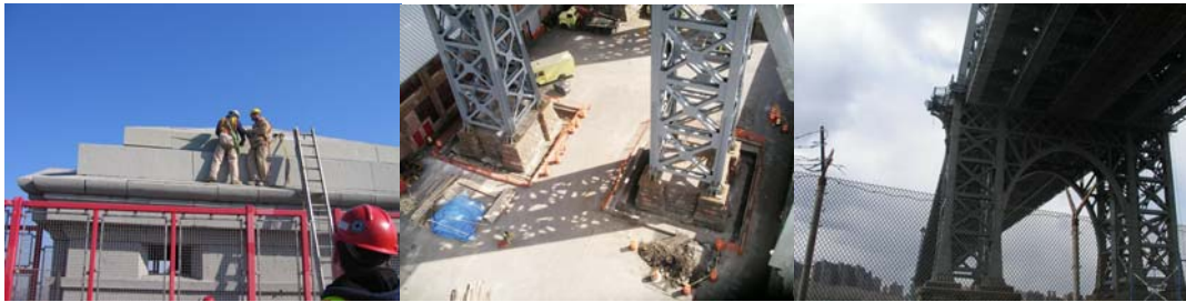
Contract #8 in 2007: Checking the Progress of the Brooklyn North Comfort Station. Seismic Retrofit Concrete Work in Brooklyn. Brooklyn Tower Balcony (South).
