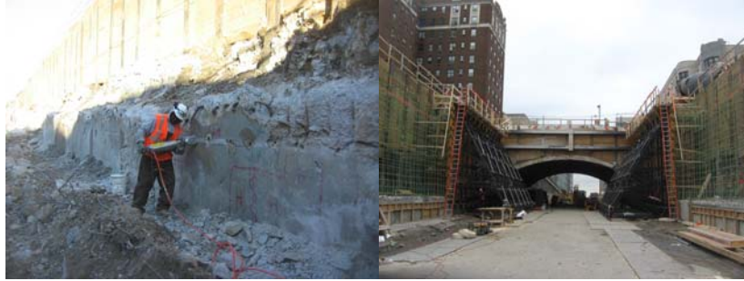
2006: Removing Concrete at the Springline of the South Abutment Stem. Formwork and Concrete Placement at South Abutment.
