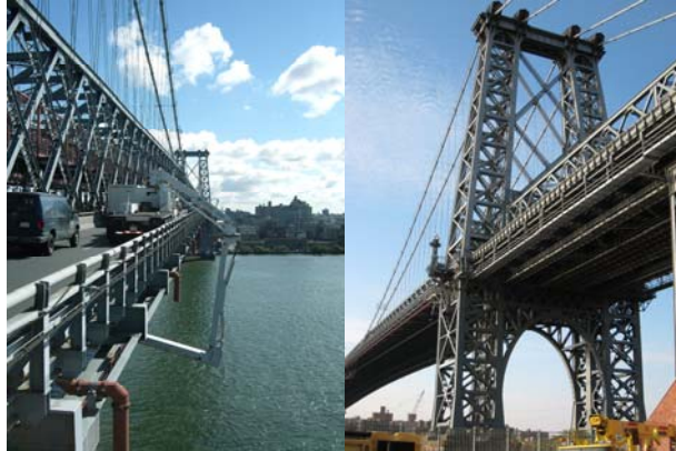
Contract #8 in 2008: Biennial Inspection of the South Roadway Under the Deck Using a Snooper Boom Truck. Brooklyn Tower in October 2008. (Tower Credit: Russell Holcomb)
