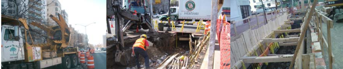
2006: Transporting Trees From East Median for Replanting. Uncovering Live ECS Cables Above Tunnel Roof Before Bridge Demolition. Excavation for Replacement of Sewer Pipes.
