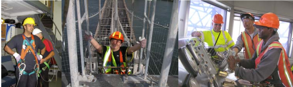
Assistant Mechanical Engineer Anatoly Orlov Checking the Harness of Mechanical Engineering Intern Shafqat Wasi. (Credit: Vera Ovetskaya) Assistant Mechanical Engineer Vera Ovetskaya Climbing to the Tower. (Credit: Gennadiy Kaplun) Construction Project Manager Gholamali Mozaffari, and Electricians Nelson Crooks and Gary Emmanuel Fixing Machinery in the Ninth Street Bridge Operator House in April 2008. (Credit: Vera Ovetskaya)
