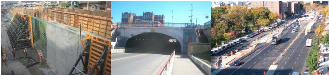
Construction of Underpass Abutment Wall. Reconstructed Grand Concourse Underpass, Sidewalks, and Bridge. Grand Concourse in November 2007.
