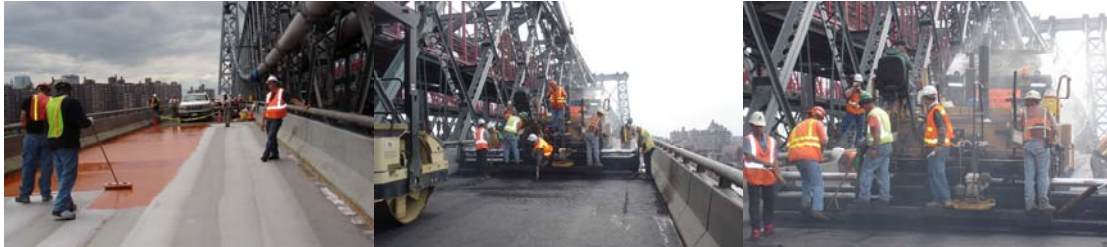
Contract #8 in 2006: Priming Application and Asphalt Paving Operation on the South Outer Roadway.
