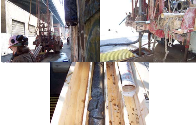
Conducting Soil Borings as Part of the Seismic Retrofit Design of the Manhattan Bridge. Drilling to a Depth of Approximately 210 Feet to Obtain an 8-foot Long Hard Rock Sample. A 2 1/2 -Foot Long Hard Rock Sample Taken From a Depth of Between 202 and 204 1/2 Feet.
