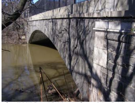
Snuff Mill Road Bridge is One of the Bridges Investigated for Scour Vulnerability and Found to be Structurally Sound, But it Remains Under Surveillance During Heavy Rains and Floods.
