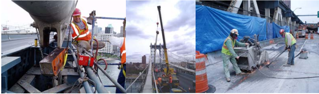
Contract #11 in 2006: Removal of Existing Suspender Rope From Cable Band on Main Span. Sawcutting Lower Roadway Deck on Manhattan Approach Span.
