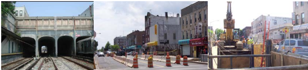
20 th Avenue Bridge in 2002. (Credit: NYSDOT) Initial Bridge Staging in May 2006. Stage I Sewer Work in 2006.
