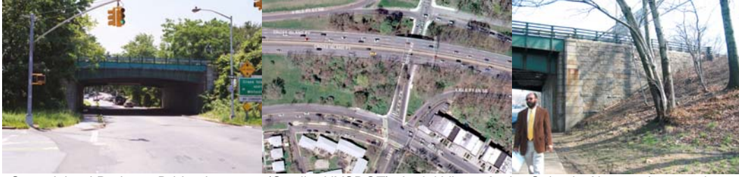
Cross Island Parkway Bridge in 2002. (Credit: NYSDOT) Aerial View. Andre Celestin About to Inspect the Abutment.
