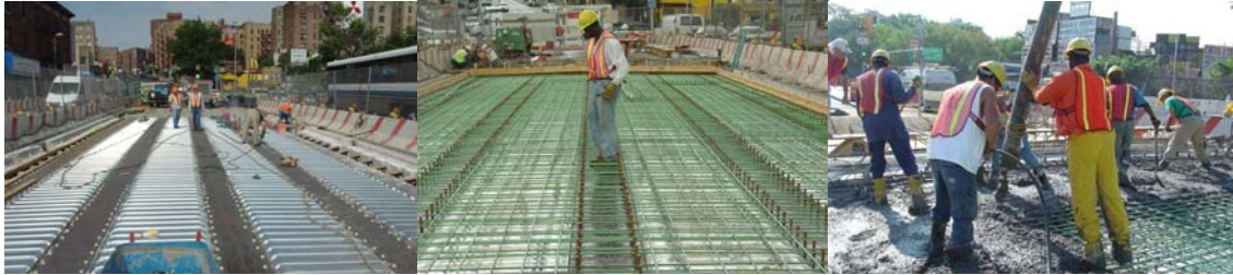
2005: Project Engineer Muhammad Siddiqui Inspecting the Stay-in-Place Formwork for the New Gun Hill Road Bridge Deck. Installing Deck Reinforcement. Concrete Placement.
