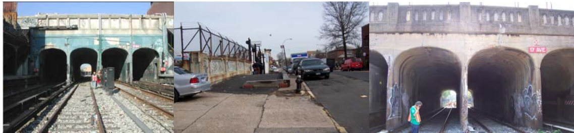
17 th Avenue Bridge in 2002. (Credit: NYSDOT) Prior to Reconstruction in 2005. Inspecting the Bridge Before Construction.
