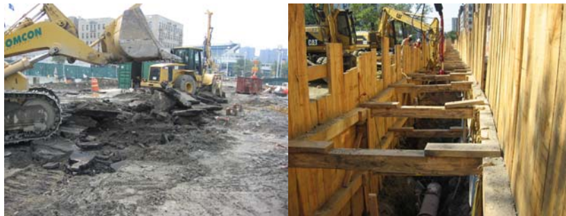
2006: Removing Asphalt and Concrete Roadway. Installing Sewer Between East 165 th and East 166 th Streets.
