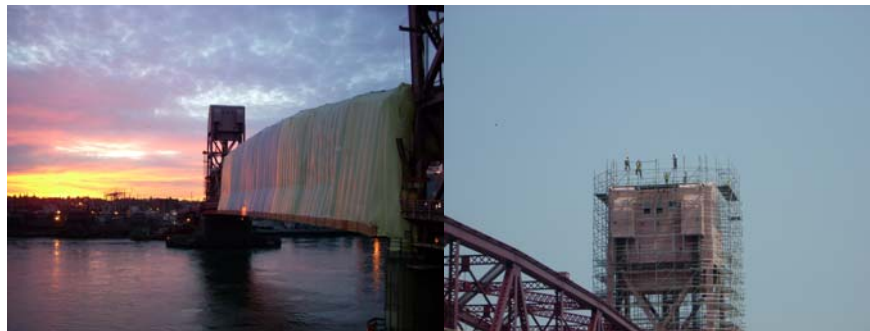
Lead Paint Removal Containment on the Lift Span in January 2008. Scaffolding Erection on the East Tower in July 2008.
