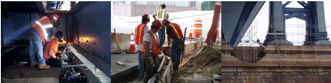
Contract #11 in 2006: Ironworkers Removing Existing Rivets in Preparation for Replacement of Lower Roadway. Installing Steel-Faced Curb for Sands Street Realignment. Erecting Scaffold to Build Painting Containment at Base of Brooklyn Tower.
