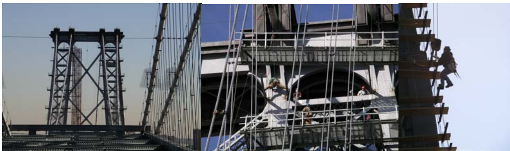
Contract #8 in 2004: Looking East at the Brooklyn Main Tower Temporary Work Platforms. Manhattan Main Tower Temporary Platform Erection. Strengthening Plate Operation on Brooklyn Main Tower.
