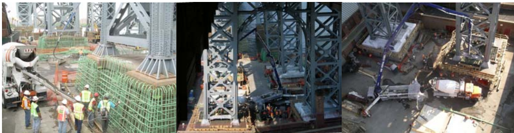
Contract #8 in 2007: Seismic Retrofit Concrete Work at the Intermediate Piers in the Kent Avenue Yard.
