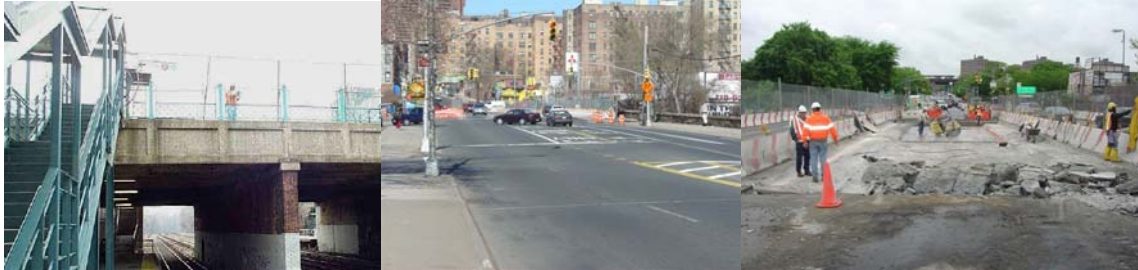
Gun Hill Road Bridge in 2002. (Credit: NYSDOT) 2005: View of Bridge at the MPT Stage. Demolition of the Existing Bridge Deck. (Deck Credit: Muhammad Siddiqui)
