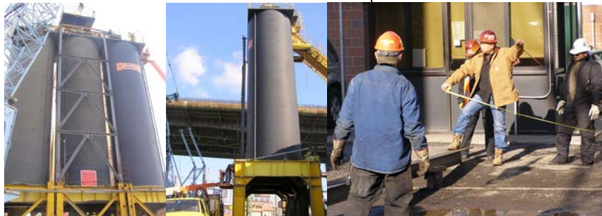
Erecting the New Support System. (Support System Credit: Hany Soliman) Measuring the Steel: Bridge Repairer & Riveters David Collins and Yiu Liu, and Assistant Civil Engineers Clara Medina (Obscured) and Hany Soliman. (Credit: George Klein)
