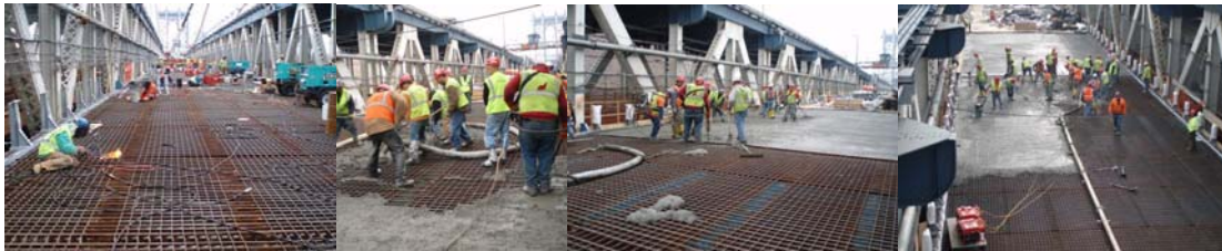
Contract #11 in 2006: Installation of Full Width Grid Deck Panels. Lower Roadway Grid Deck Concrete Pour in December 2006.
