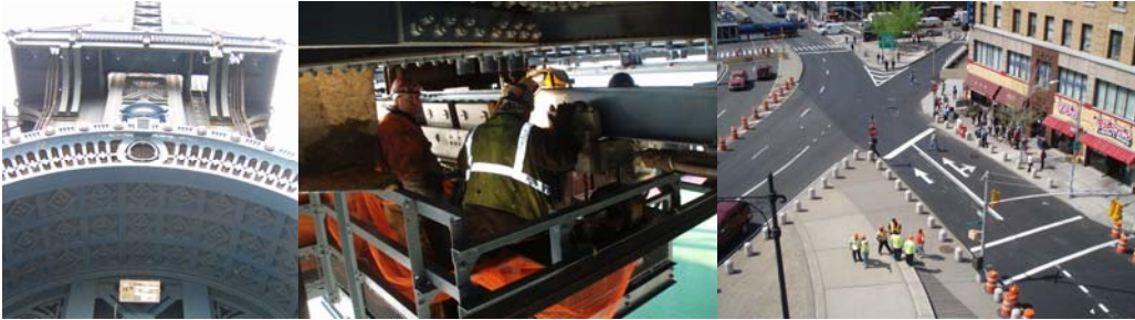
Contract #11 in 2008: Renovated Tower Canopy. (Credit: Peter Basich) Rehabilitating the Maintenance Traveler Platforms. Striping for the New Traffic Pattern in Manhattan Plaza.
