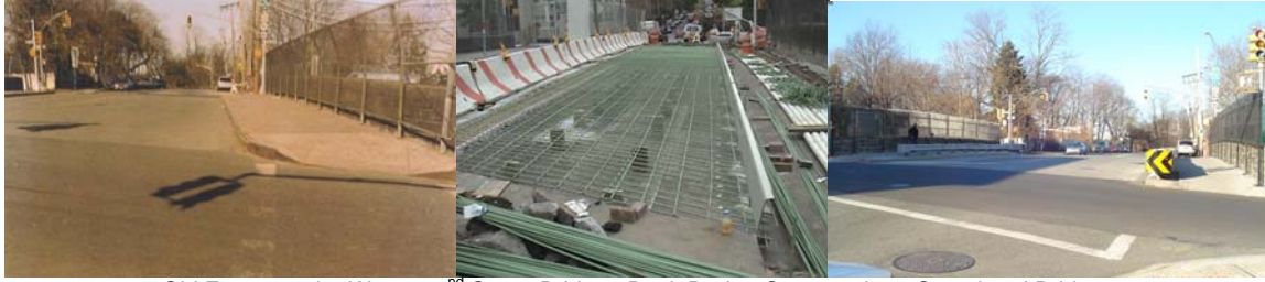
Old Fence on the West 232 nd Street Bridge. Deck During Construction. Completed Bridge.
