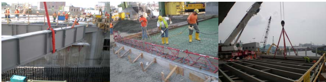
Installation of New Hamilton Avenue West Bridge Structural Steel, and Placement of Concrete for the New Northwest Sleeper Slab in July 2008. Installation of New Southwest Sidewalk in August 2008.
