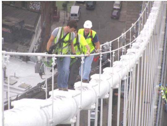
On September 8, 2008, Researchers From Columbia University and Engineer-In-Charge Brian Gill (at Right) Climbed the Manhattan Bridge and Installed Accelerometers and GPS Sensors to Monitor the Overall Dynamic Behavior of the Bridge to Improve Computer Modeling Techniques for a Possible Reduction of Seismic Retrofit Modifications. (Credit: Bojidar Yanev)
