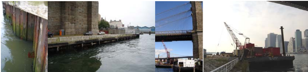
Holes in the Steel Sheet Cofferdam of the Brooklyn Bridge Esplanade in April 2007. View of the Work Area in October 2007. The Barge and Equipment Used on the Steel Cofferdam Repairs. (Credit: Thomas Leung)
