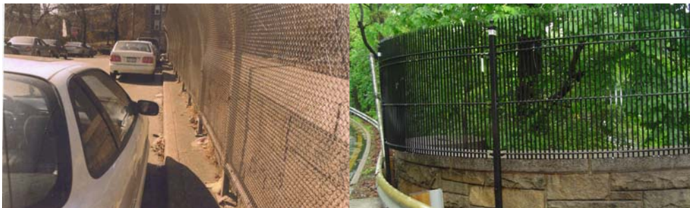
Old Fence on the Manhattan College Parkway Bridge. Newly Installed Picket Fence.
