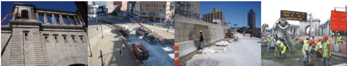
Contract #11 in 2007: Masonry Cleaning of the Upper Section of the South Face of the Manhattan Anchorage. Milling of the Existing Lower Roadway Pavement at the Manhattan Plaza. Masonry Cleaning of the Lower Roadway Wall at the Brooklyn Transition. Concrete Placement in Manhattan Plaza at the Entrance to the Lower Roadway.
