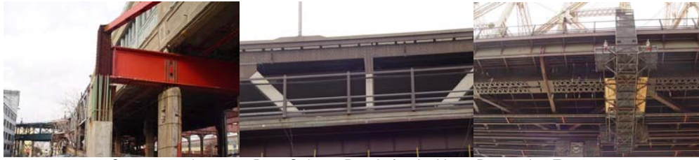
Contract #6 in 2005: Bent Column Ready for Jacking. Decorative Fence. Repairing the Drainage Pipes.
