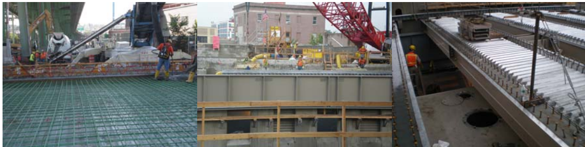
Placement of New Concrete on the Hamilton Avenue Southwest Approach Slab, Installation of New West Bridge Structural Steel, and Installation of New West Bridge Deck and Counterweight in July 2008.
