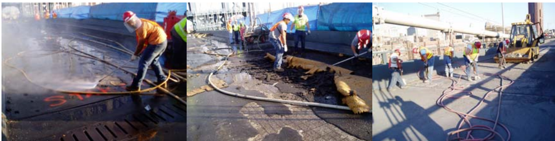
Contract #11 in 2005: Waterblasting to Remove Existing Microsurfacing From the South Upper Roadway. Manually Removing the Microsurfacing.
