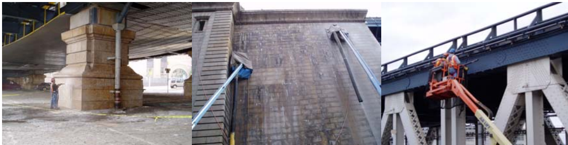
Contract #11 in 2005: Masonry Cleaning of the Brooklyn Granite Pier and of the North Face of the Brooklyn Anchorage. Installing Conduit for the New North Upper Roadway Street Lighting.
