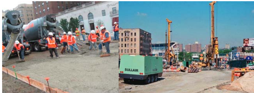
2007: Pouring Concrete for Pavement. Rigs in Lou Gehrig Plaza Drilling and Installing Cantilever Soldier Piles.
