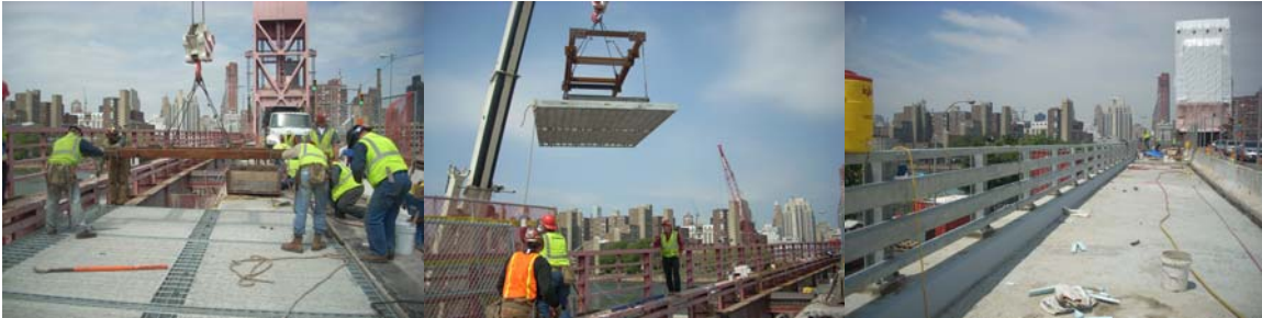
Concrete Filled Grid Deck of the Queens Approach in April and May 2008. Stage I Roadway Construction of the Queens Approach in July 2008.
