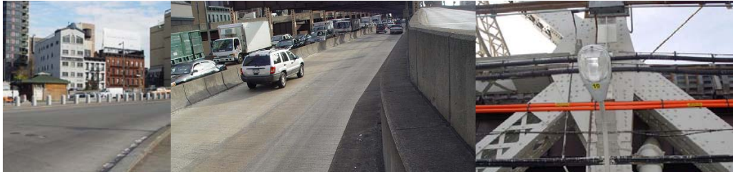
Contract #6 in 2005: Manhattan Plaza Bollards. Full Width Deck Repair on South Inner Roadway. New Luminaire on North Upper Roadway.
