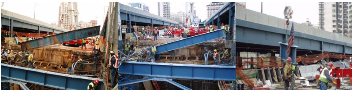
2007: Removal and Replacement of the Final Existing Manhattan Bridge Lower Roadway Floorbeam.
