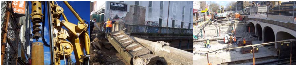
Removing the 20 th Avenue Bridge Arch Overburden in January 2007. Bridge demolition in February 2007.
