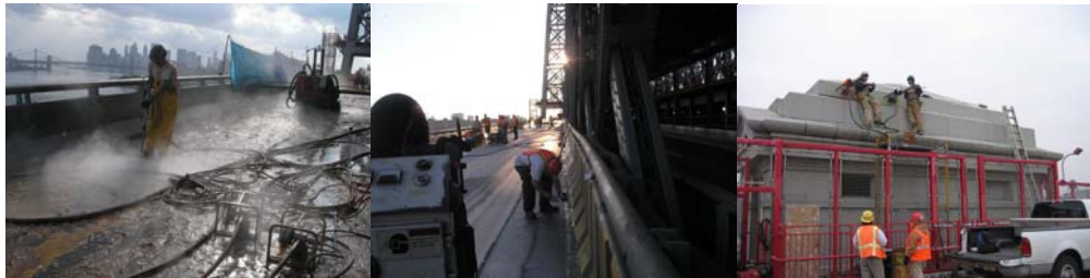
Contract #8 in 2006: Water Blasting. Curb Angle Cleanup and Tack Coat. Core Drilling The Brooklyn North Comfort Station.
