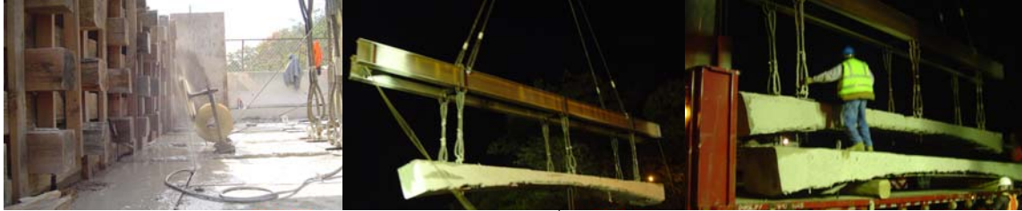
2006: Cutting and Removing the Existing West 252 nd Street Bridge Sections Over the Parkway.
