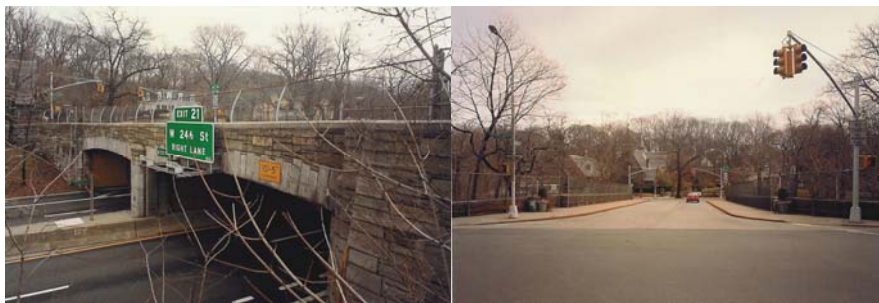
West 252 nd Street Bridge Before Reconstruction.
