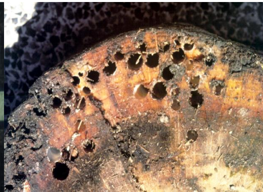
Teredo Damage (holes up to ¼" diameter)
