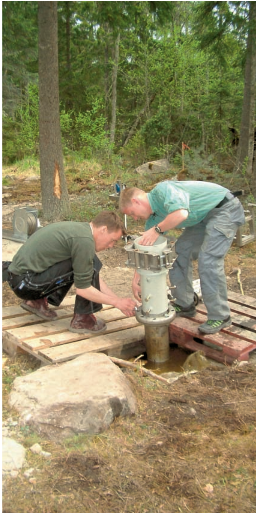
Site investigations, i.e. thorough investigations of the bedrock from the ground surface, are being conducted in the municipalities of Östhammar and Oskarshamn.
