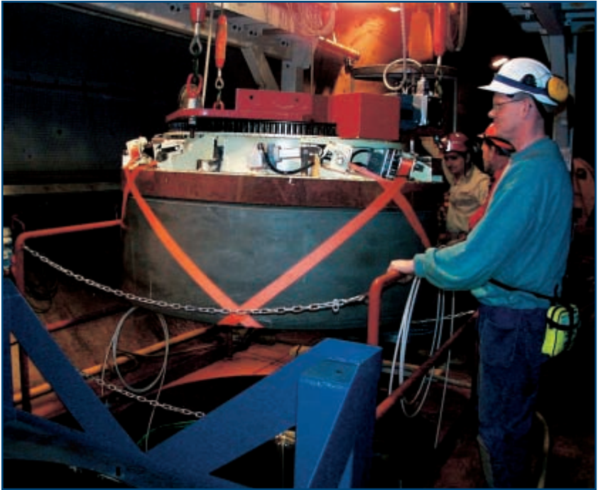
Each deposition hole is lined with blocks and rings of bentonite. Here a block is lifted into place.
