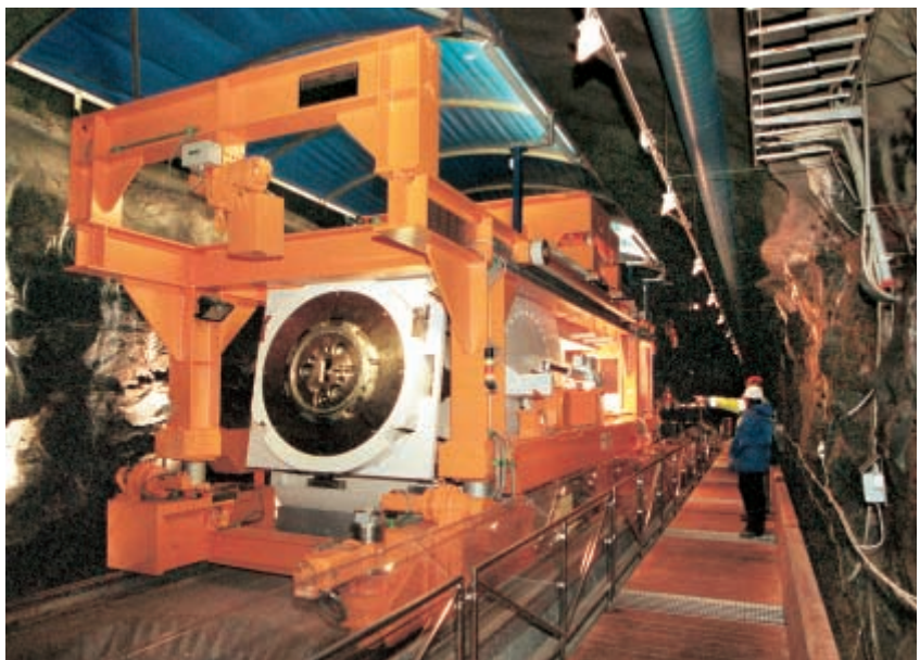
The canisters are placed in the deposition holes with the aid of a specially-built machine.
