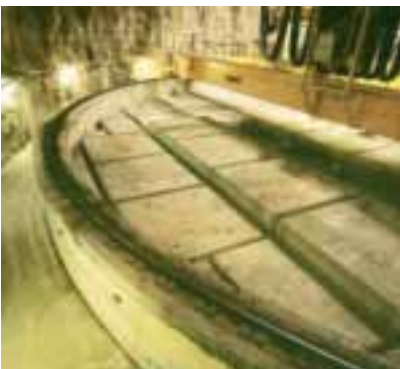
Most of the radioactivity in the facility is present in the silo.
