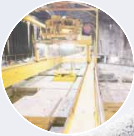
2 Casks with intermediate-level waste are carried to the top of the silo by overhead crane. The silo is divided into shafts into which the casks are lowered.
