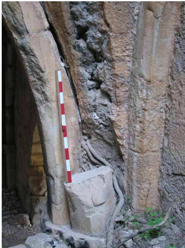
1. Damage caused by vegetation in the guesthouse below the castle.
