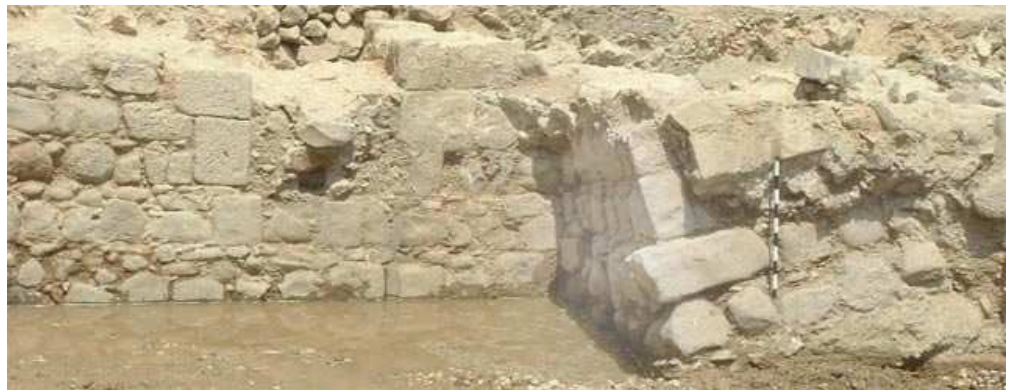
7. Walls from the Byzantine–Umayyad periods; the wall on the right was damaged by the earthquake.
