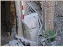
1. Damage caused by vegetation in the guesthouse below the castle.
