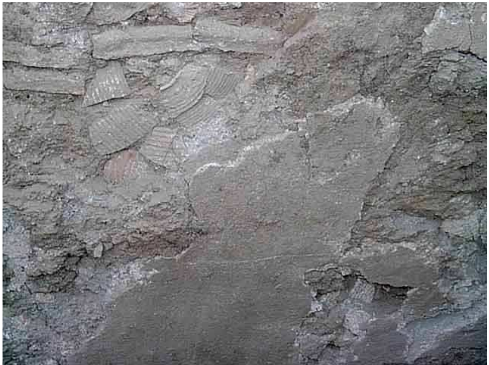
6. Plaster remains and the potsherd base layer on the reservoir's wall, looking west.
