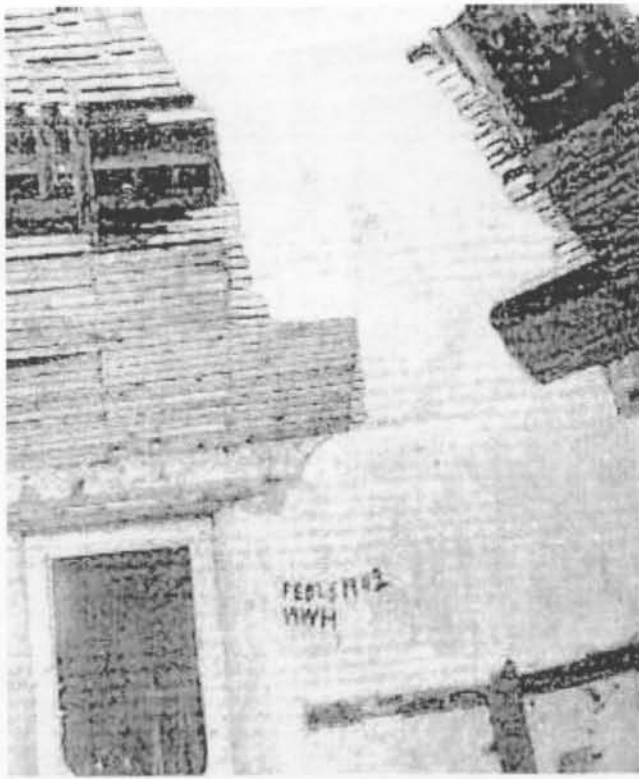
Here is the ceiling area that needed new lath and plastering. Wonder if HWH was about to go off to war on February 28, 1942.
