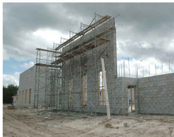
Construction on the new 37,000 square foot library is currently under way, and expected to be finished in 2011.
