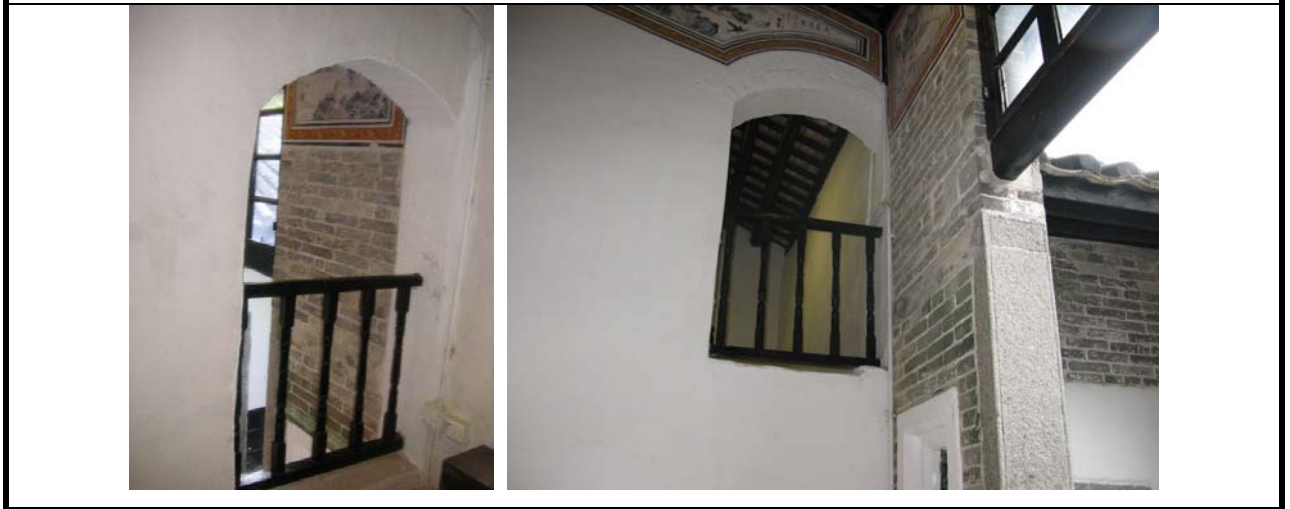
2.11) Arch openings with wooden balustrade at the cockloft of the rear side rooms
