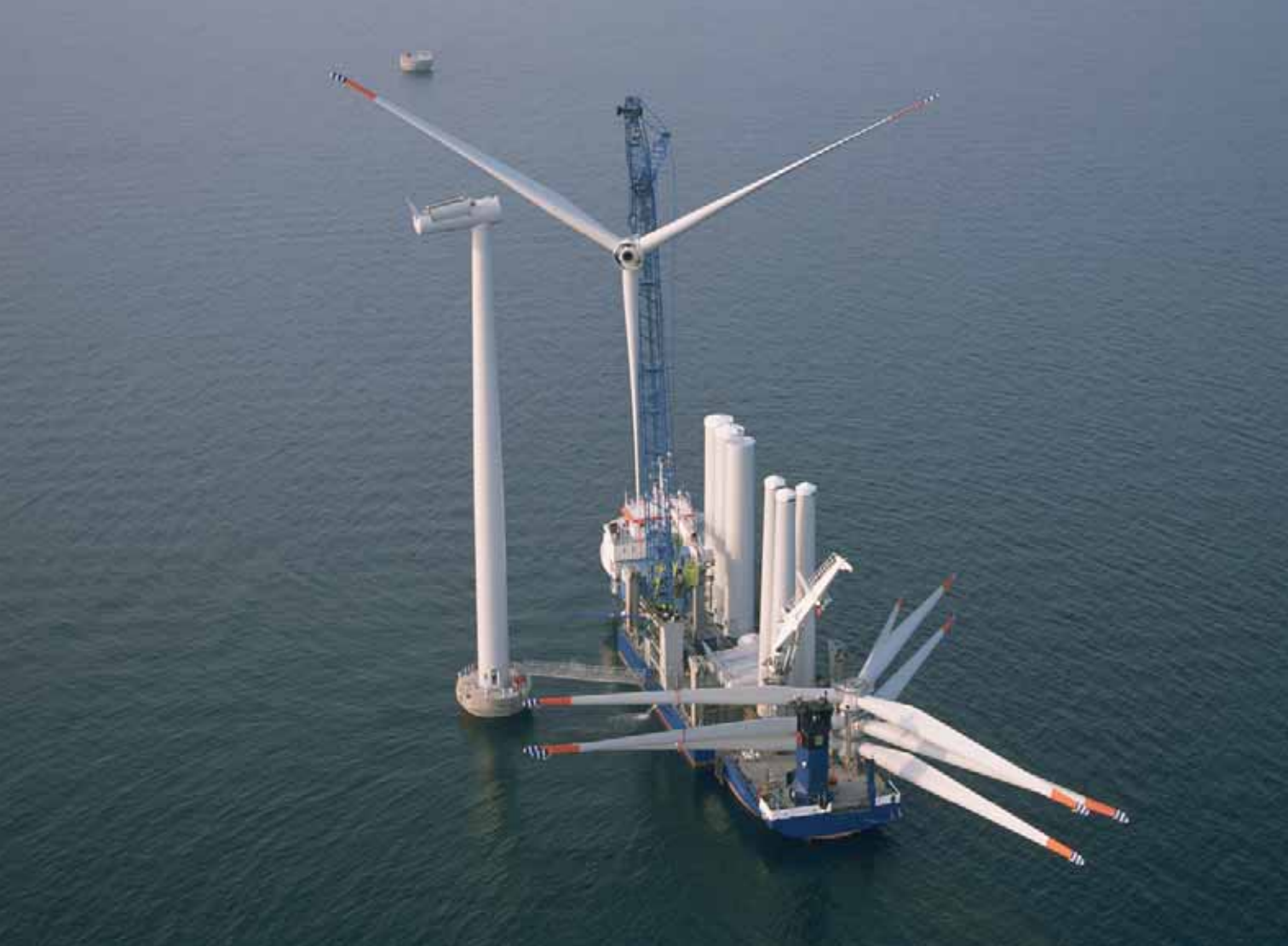
FIGURE 3.9 Construction of the first wind turbine at Nysted Offshore Wind Farm PHOTO: NYSTED OFFSHORE WIND FARM
