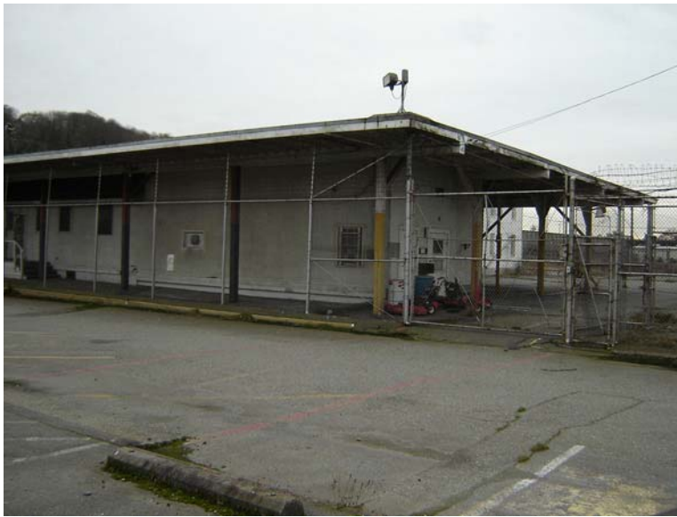
View of the southeast corner of Building #218 (Mess Hall) below Building #275 (Assembly Shed)
