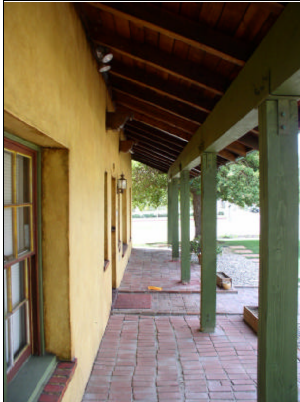
Front entry porch along north elevation with overhang, posts, and exposed beams, looking west
