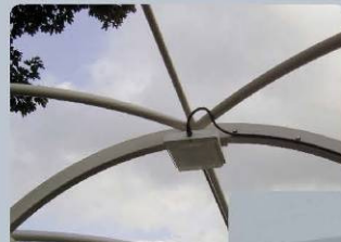
Example of Bridge Lighting
