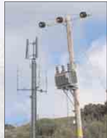
Electricity and mobile phone masts
